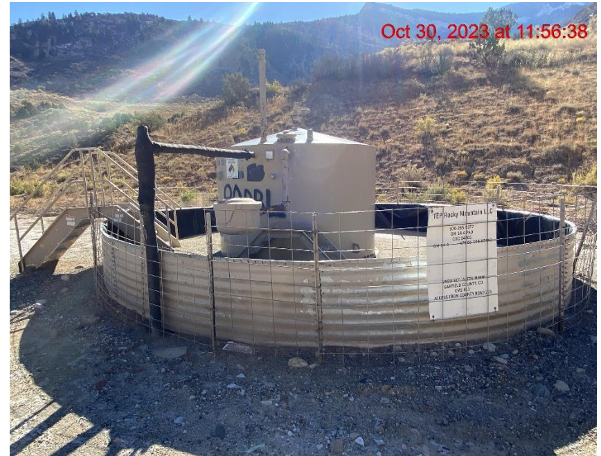
Tank Battery – Photo #07244
