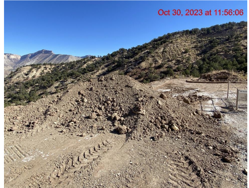
Unprotected Soil Stockpile – Photo #07242
