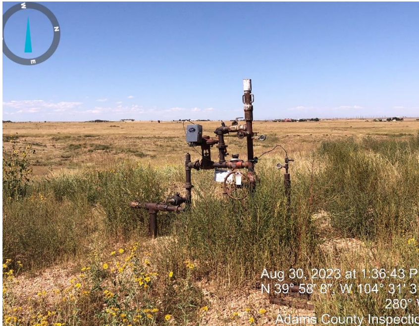
Photo #1 Well head.
