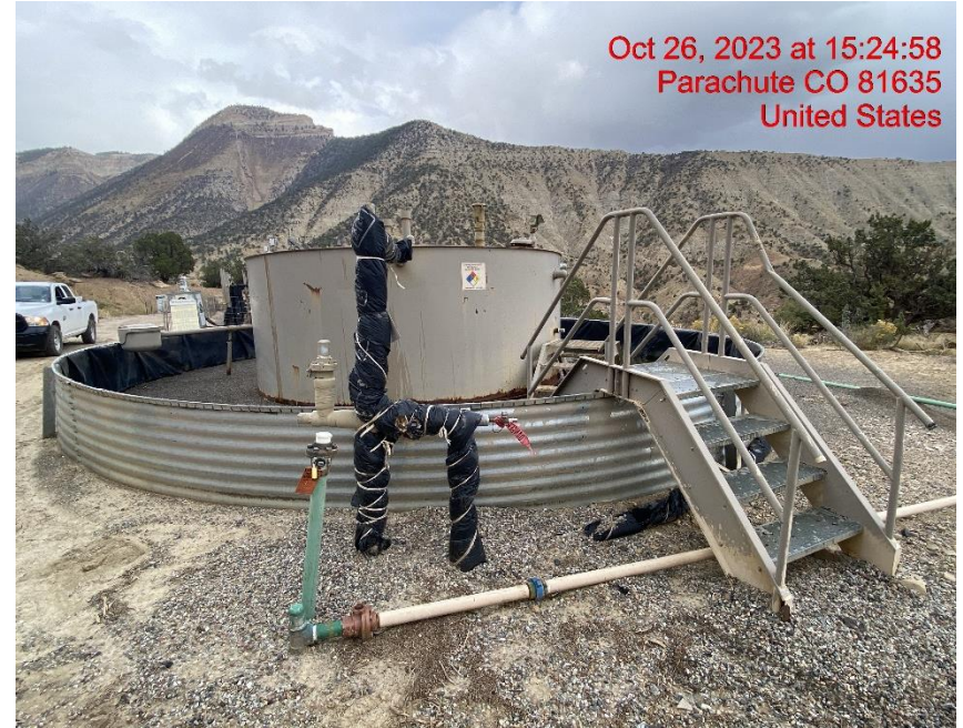
Tank Battery – Photo #07194
