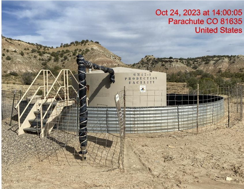
Tank Battery – Photo #07138
