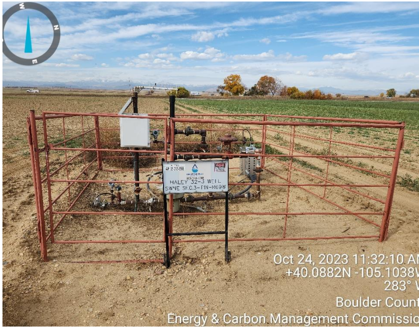
Photo 1 well head and equipment
