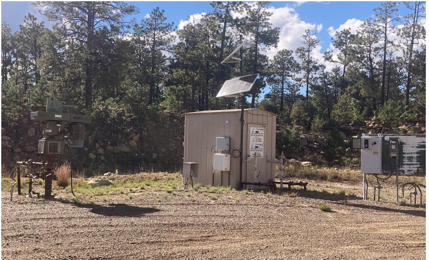
PHOTO 3: V WELLHEAD AND EQUIPMENT
