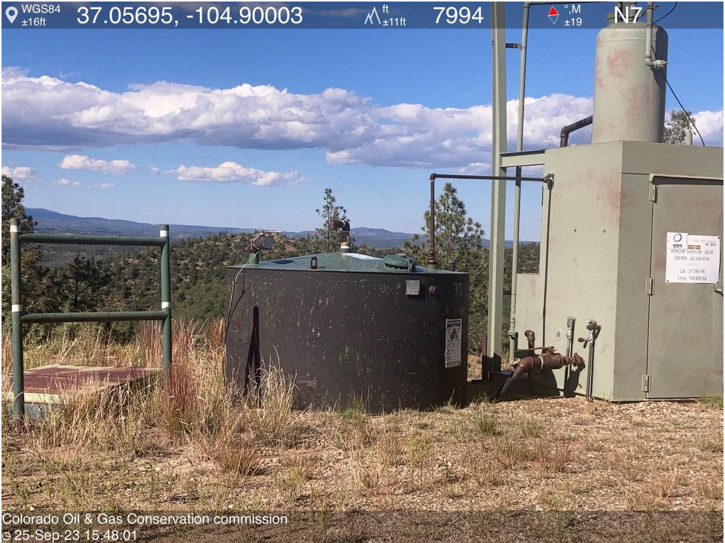
PHOTO 4: 30 BBL PRODUCED WATER TANK.
