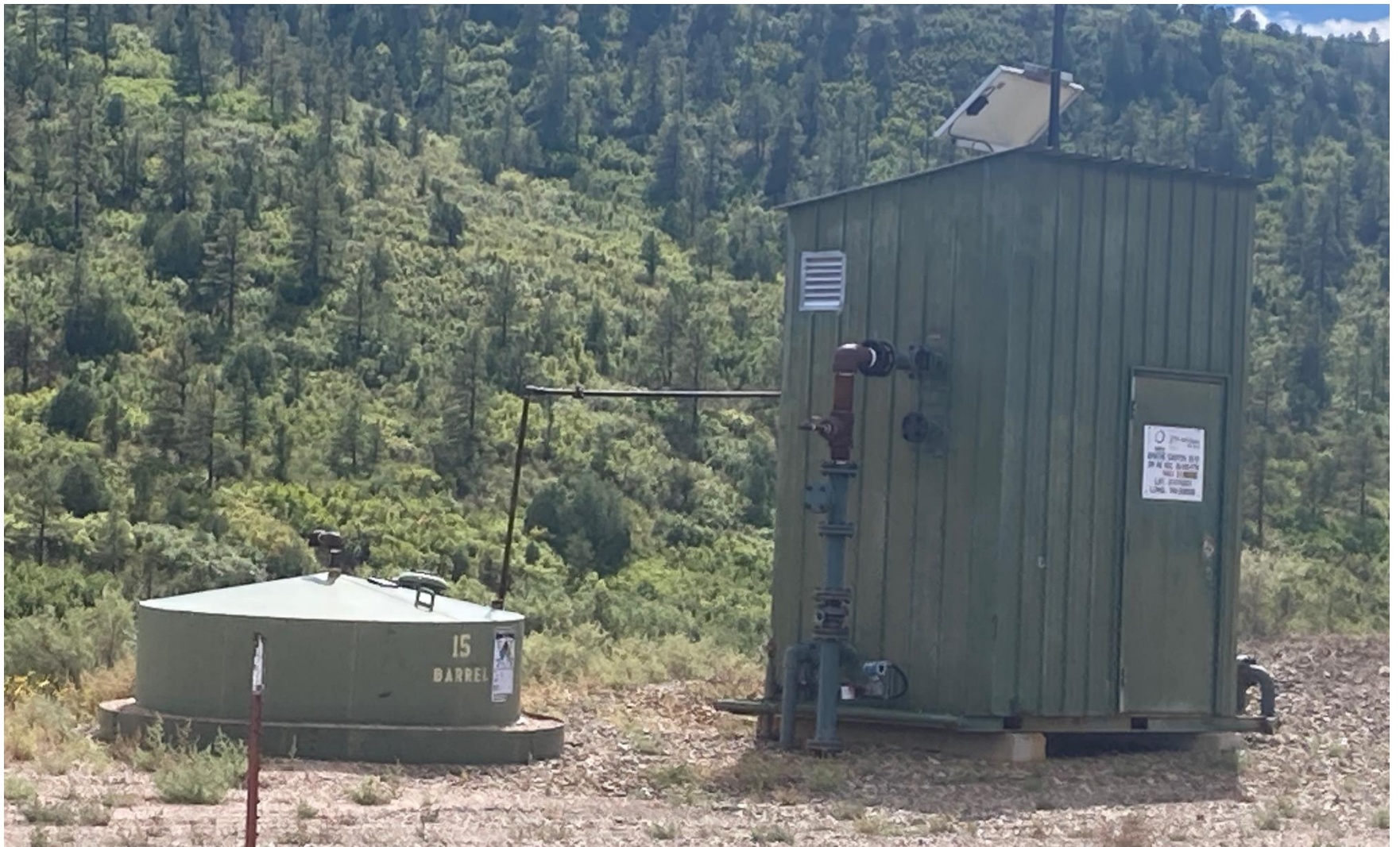
PHOTO 3: WELLHEAD AND EQUIPMENT
