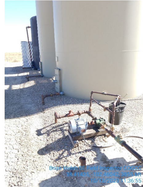
North side of tank battery and circulating pump with catch basin
