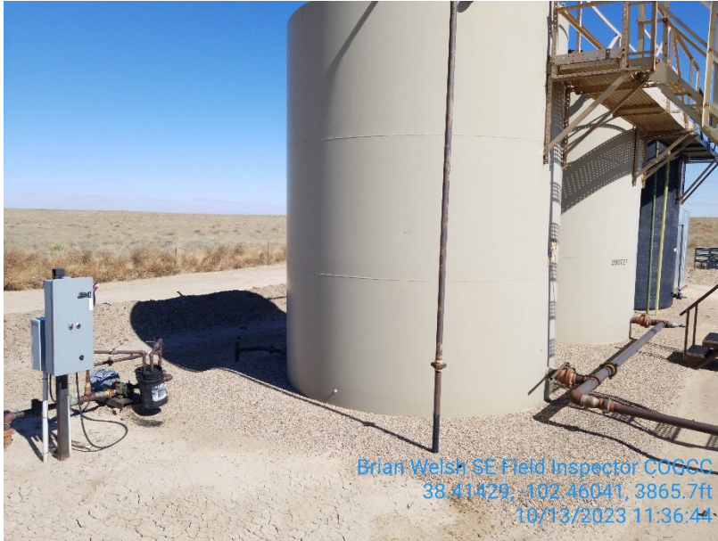
South side of tank battery
