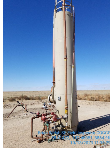
Treater with pipe hanging from the top
