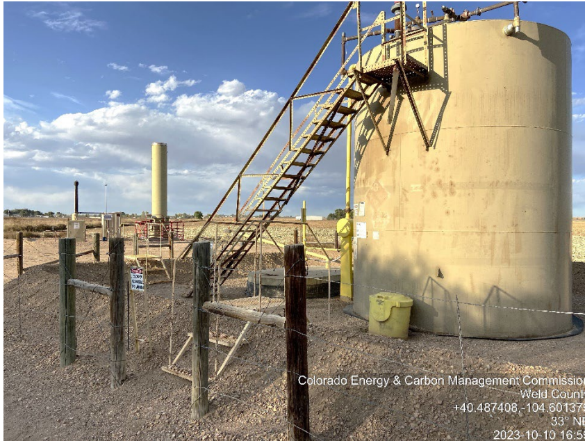
Photo #1 Heldt 12-18 Battery site Active
