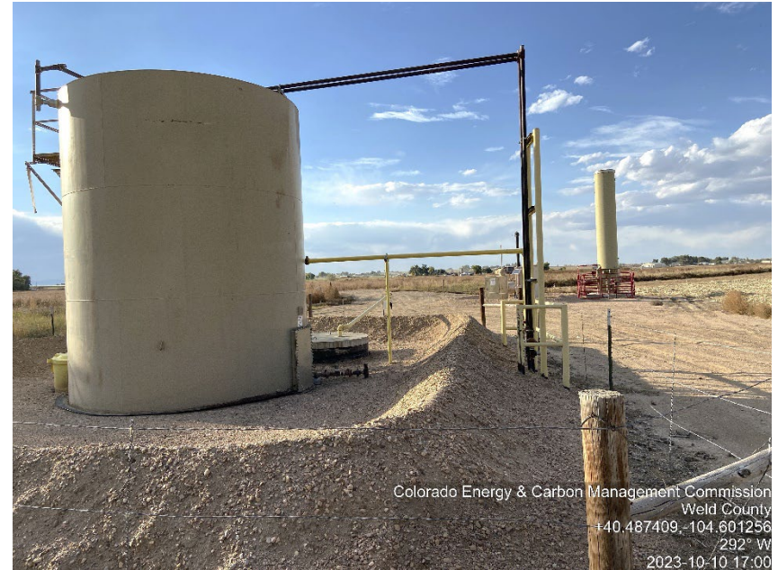
Photo #2 Heldt 12-18 Battery site Active Tank(s): SE corner
