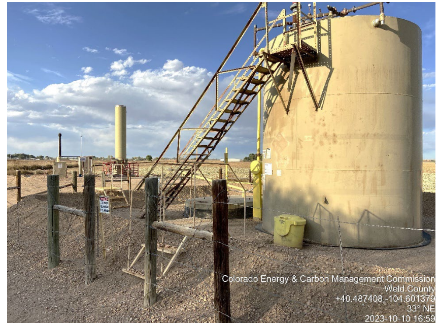
Photo #2 Heldt 12-18 Battery site Active Equipment Documented; Loc ID: 330743
