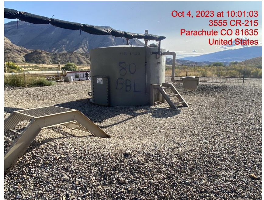
Tank Battery – Photo #06742
