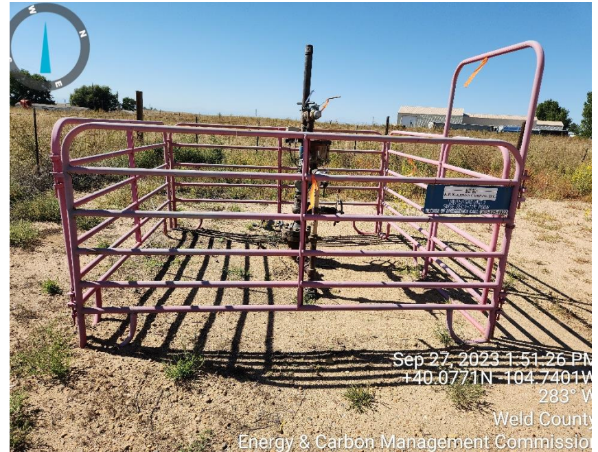
Photo 2 well head and equipment
