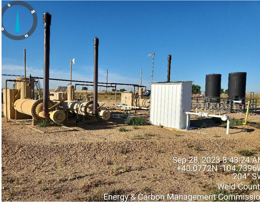
Photo 5 production equipmenr and meter run
