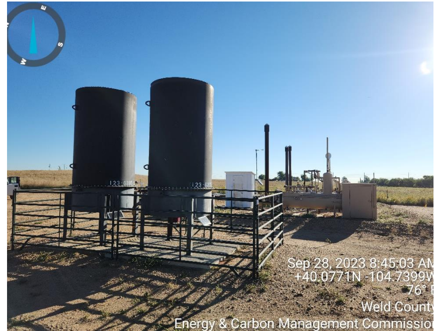
Photo 8 ECD's and production equipment
