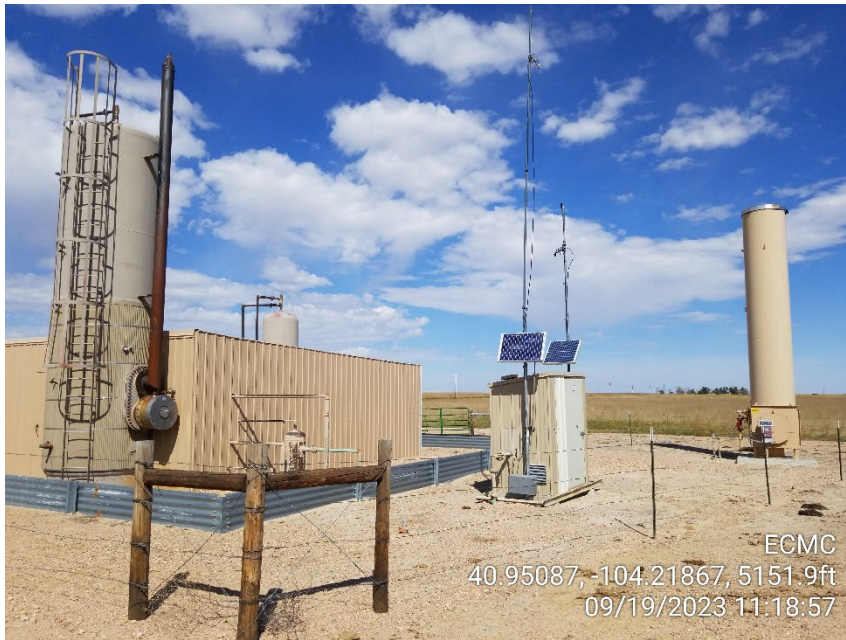
Photo 3 – Heater Treater, Gas Meter and ECD
