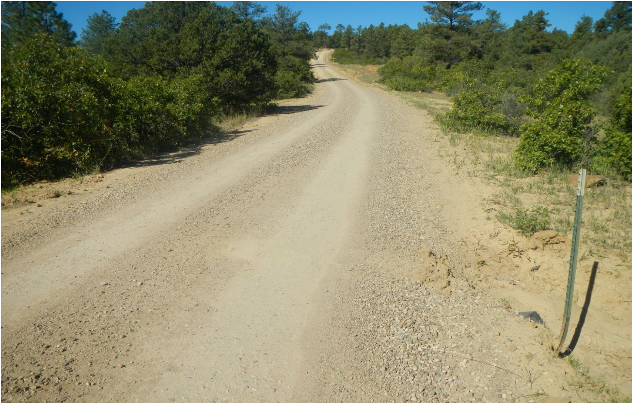
Photo 2. Facing northwest along the main road. Additional gravel has been applied to areas of the road.
