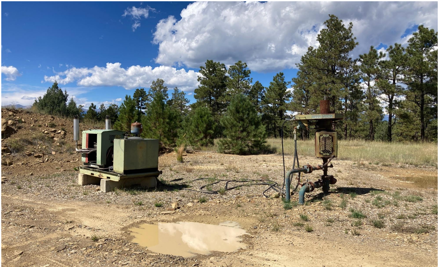
PHOTO 3: WELLHEAD AND EQUIPMENT
