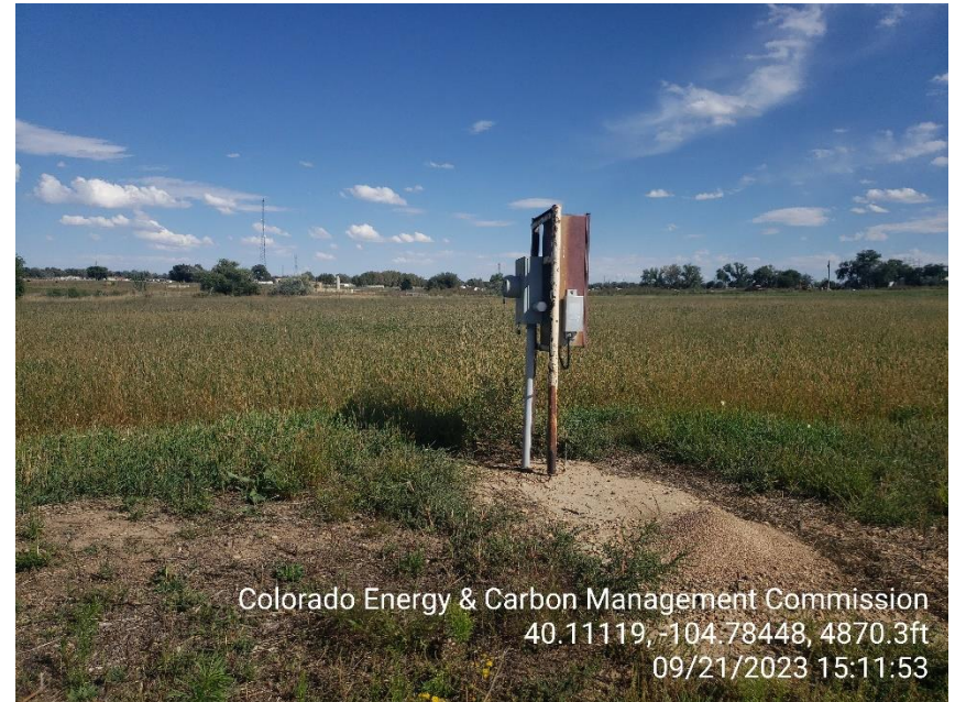
Photo 4 electric panel, meter box.
