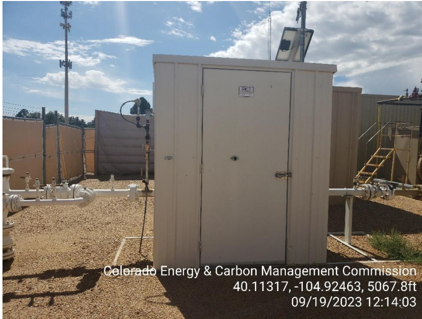
Photo 3 Gas Meter Run.
