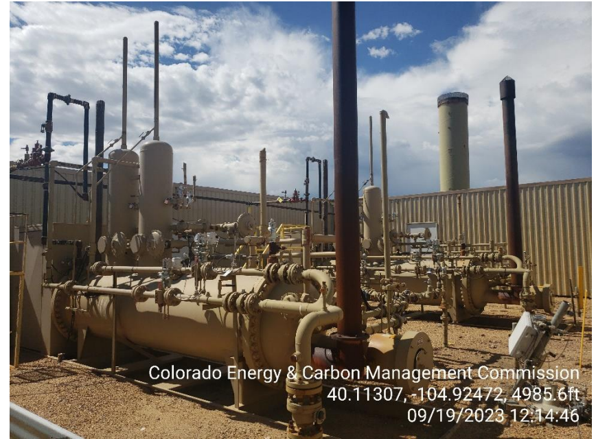
Photo 4 Horizontal Heated Separators.
