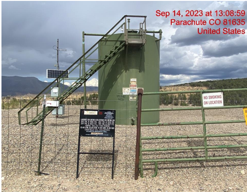
Tank Battery – Photo #06423
