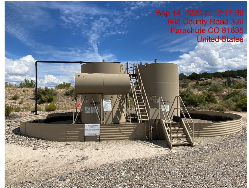
Tank Battery – Photo #06411
