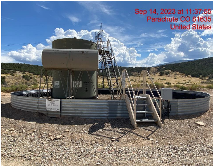
Tank Battery – Photo #06396
