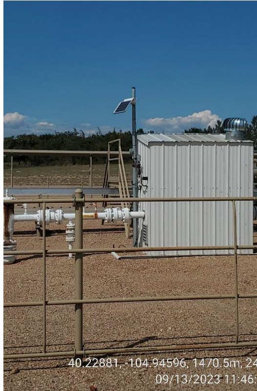
Photo 2 GMR and Pig Station
