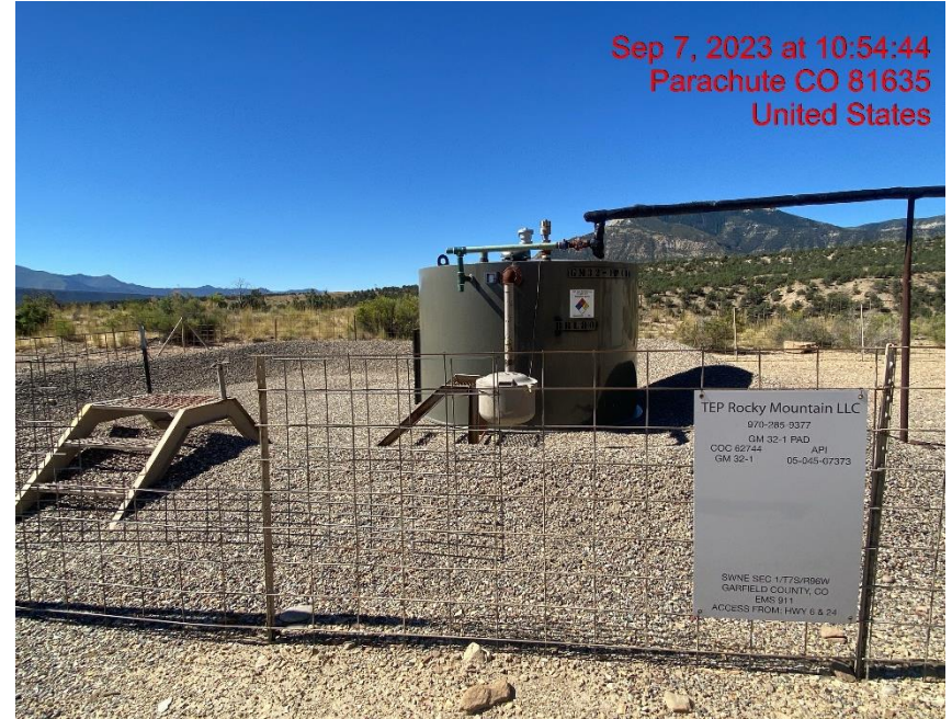
Tank Battery – Photo #06303
