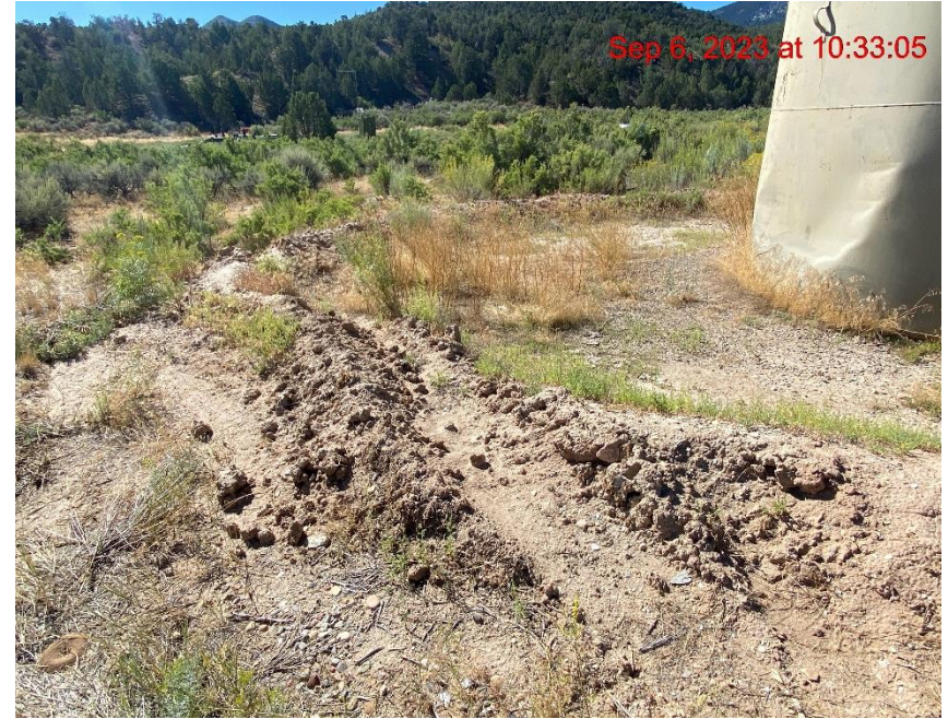
Secondary Containment Berm Damaged – Photo #06290
