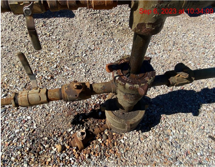
Stuffing Box Leak/Stained Soil – Photo #06295
