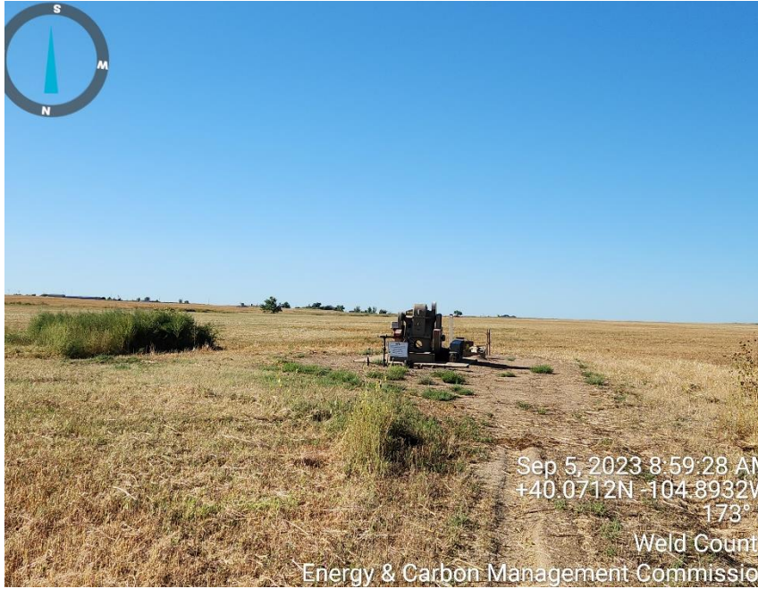
Photo 1 well head and equipment
