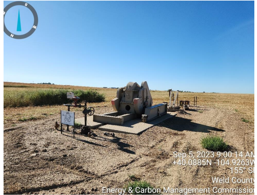
Photo 2 well head and equipment
