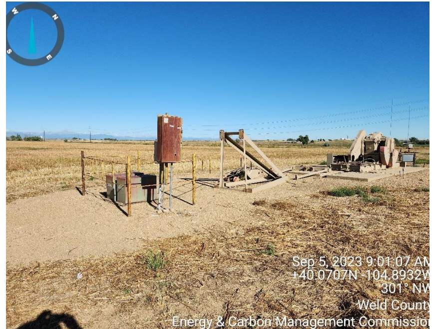
Photo 4 electrical panel and equipment
