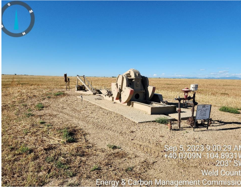
Photo 3 well head and equipment
