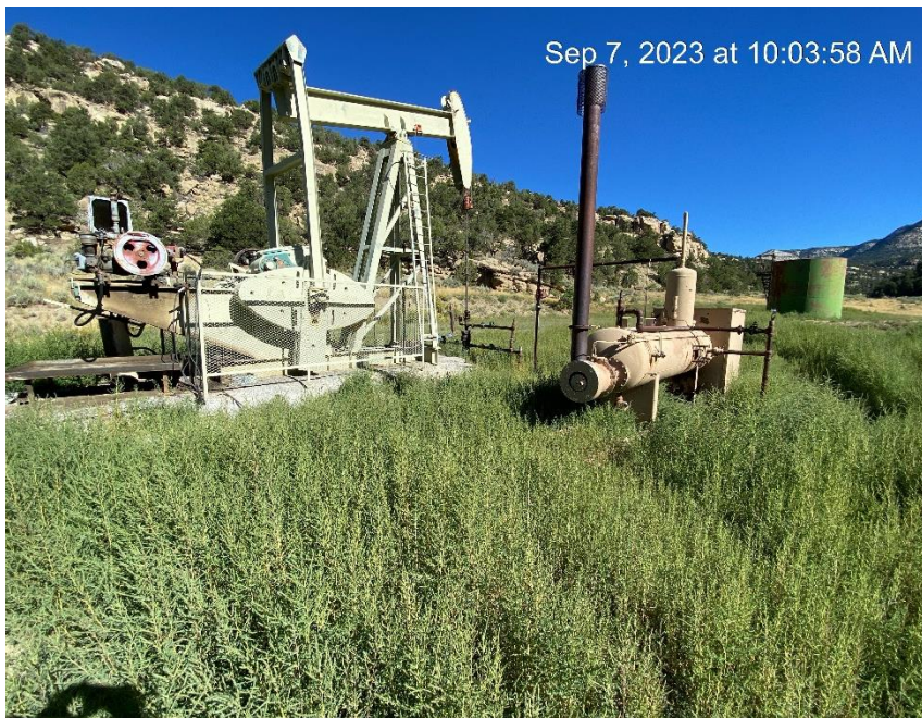
Pumping unit and separator
