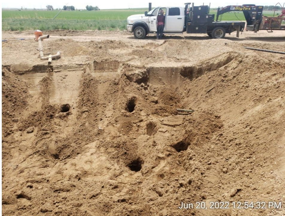
#5C - UPRC-65N64W 23SESW – Southern Sidewall of Western Produced Water Vessel Excavation – WPWVS01@6.0’– No Impacts Noted – PID 0.3ppm – Facing South
