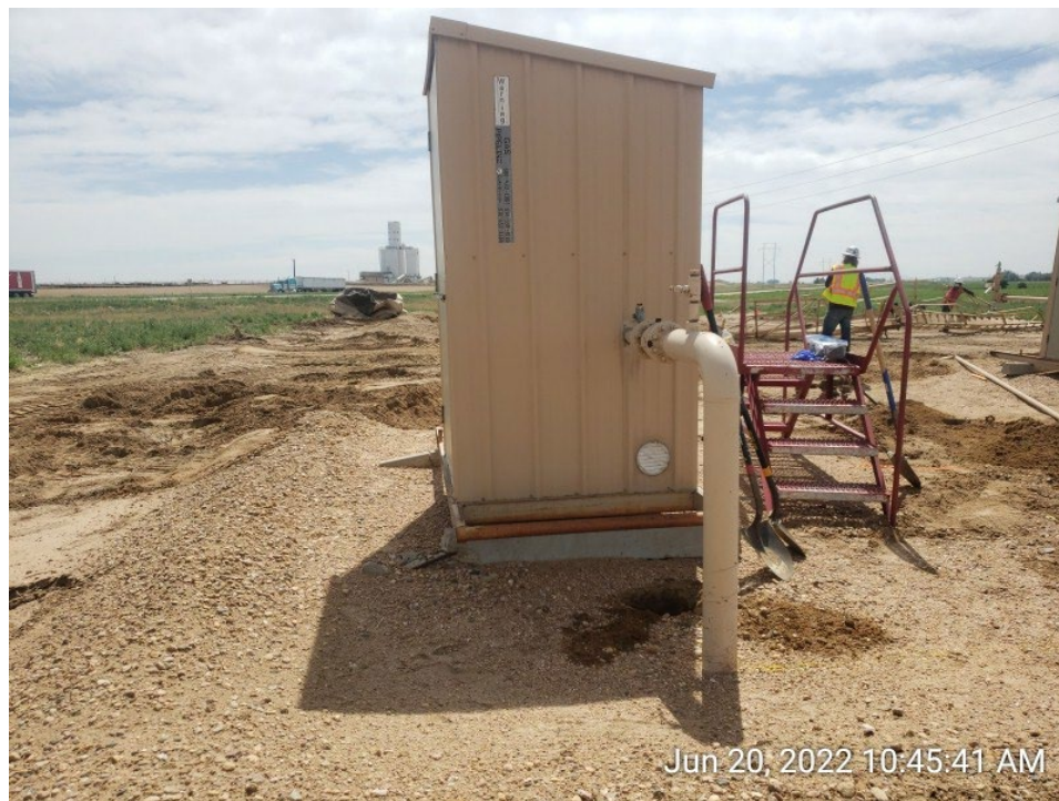
#10A - UPRC-65N64W 23SESW – Northern Third-Party Meter Shed – MET01@6.0” – No Impacts Noted – PID 1.3ppm – Facing East
