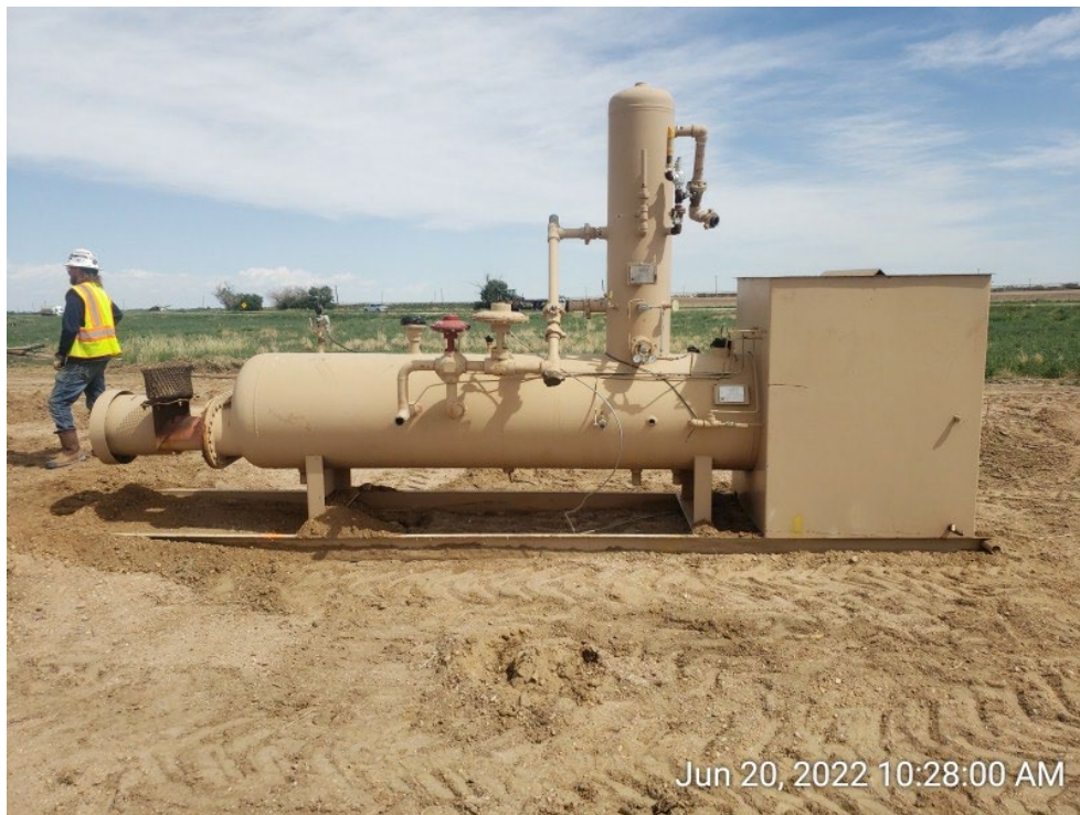
#7A - UPRC-65N64W 23SESW – Separator – Good Condition – Little to No Corrosion – Facing North
