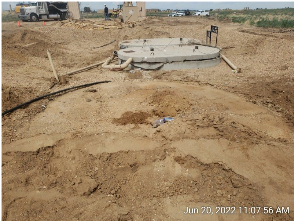
#2A - UPRC-65N64W 23SESW – Western Above Ground Storage Tank – WAST01@6.0” – No Impacts Noted – PID 0.1ppm – Sample Submitted for Lab Analysis – Facing West
