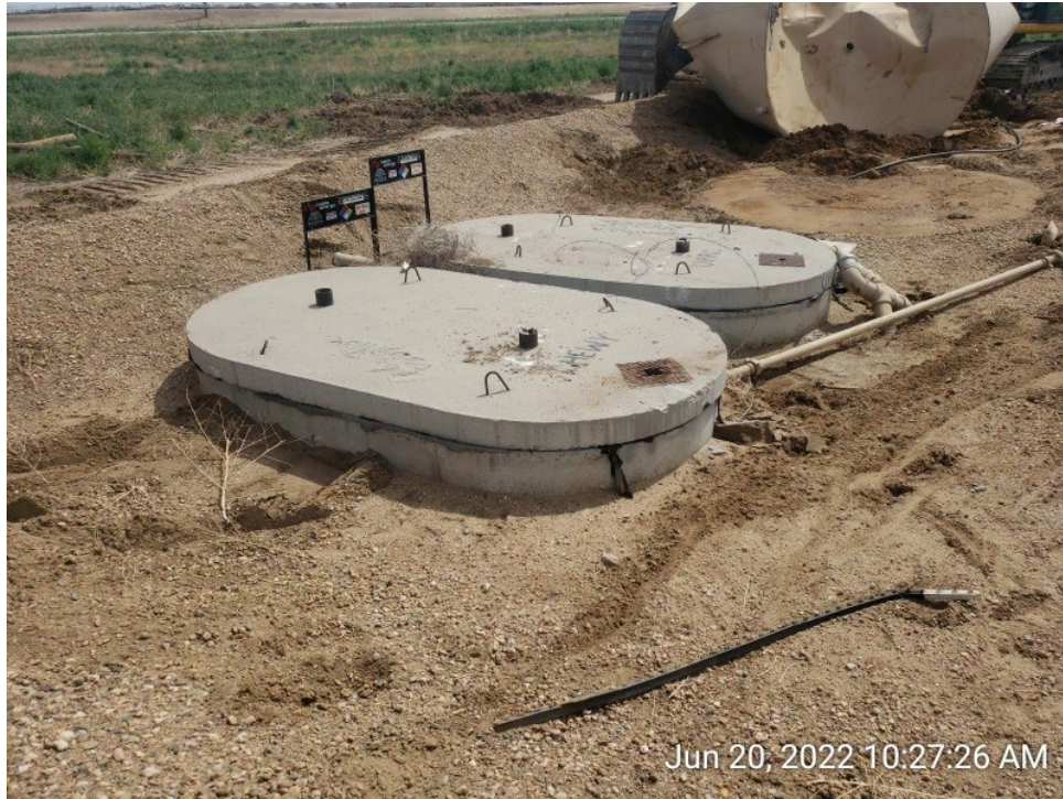
#3A - UPRC-65N64W 23SESW – Produced Water Vessels – Good Condition – Little to No Corrosion – Facing Northeast
