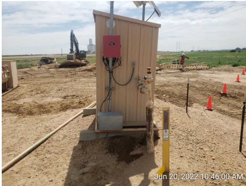
#11A - UPRC-65N64W 23SESW – Northern Third-Party Meter Shed – MET02@6.0” – No Impacts Noted – PID 0.2ppm – Facing East
