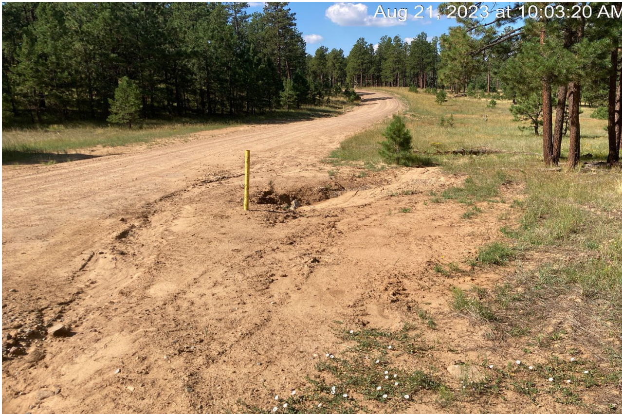
Photo 5. Facing southeast at Lat/Long:37.01055,-104.89653. A culvert was installed at this area of the road. Disturbed soils need to be seeded and stabilized.
