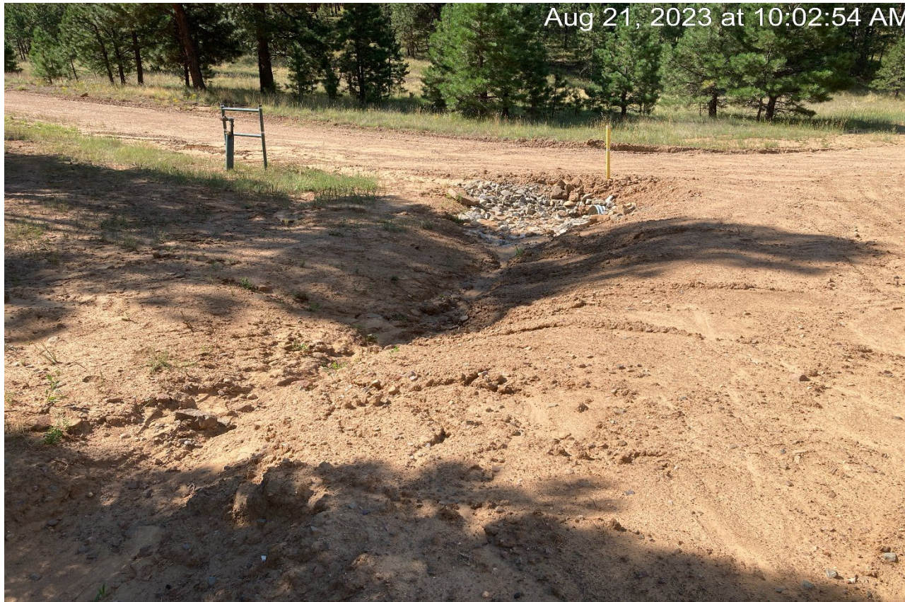
Photo 4. Facing southeast at Lat/Long: 37.01055, -104.89653. A culvert was installed at this area of the road. Disturbed soils need to be seeded and stabilized.
