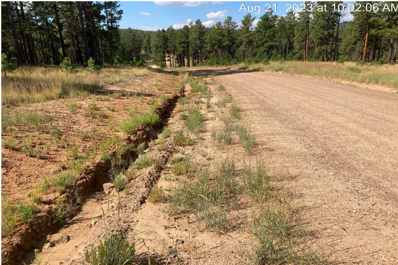
Photo 3. Facing south along the main access road. This area was graded and vegetation is establishing. Additional BMP's such as check dams may be needed to prevent erosion.
