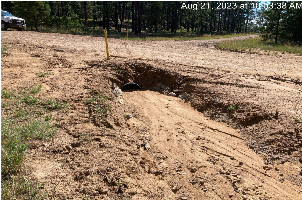
Photo 6. The culvert outlet is half full of sediment and needs to be cleaned out. A sediment trap could be beneficial to contain erosion.
