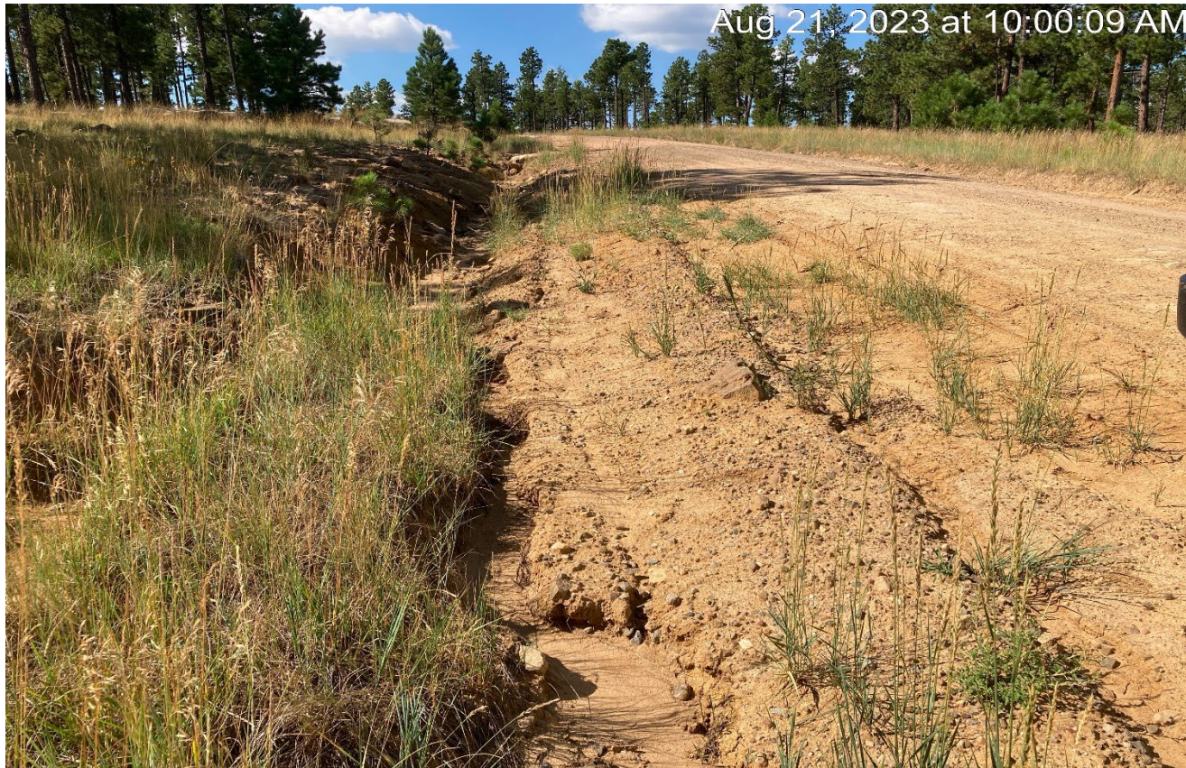
Photo 1. Facing southwest along the main access road at Lat/Long: 37.01620,-104.89531. There is erosion along this area which needs to be controlled.
