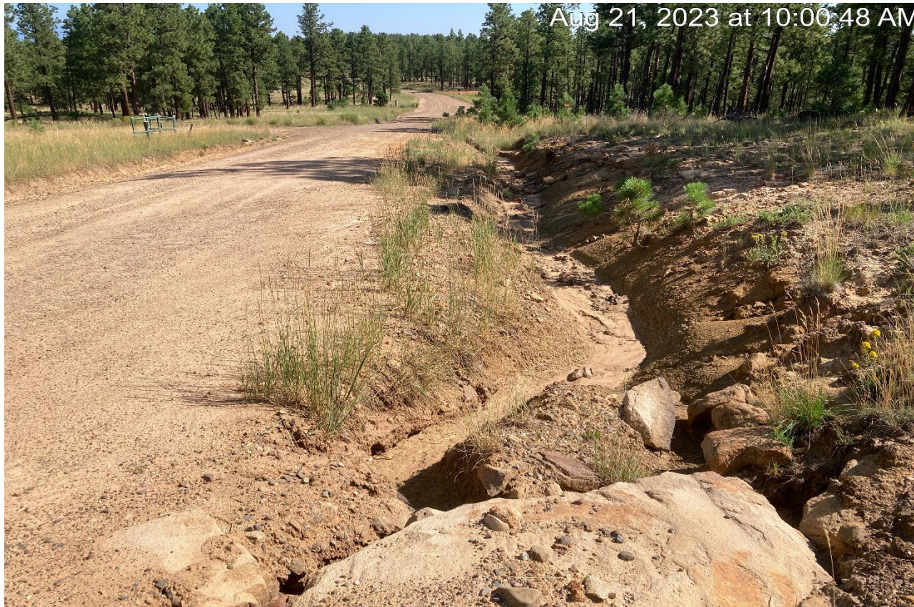
Photo 2. Facing northeast along the main access road at Lat/Long: 37.01620,-104.89531. There is erosion along this area which needs to be controlled.
