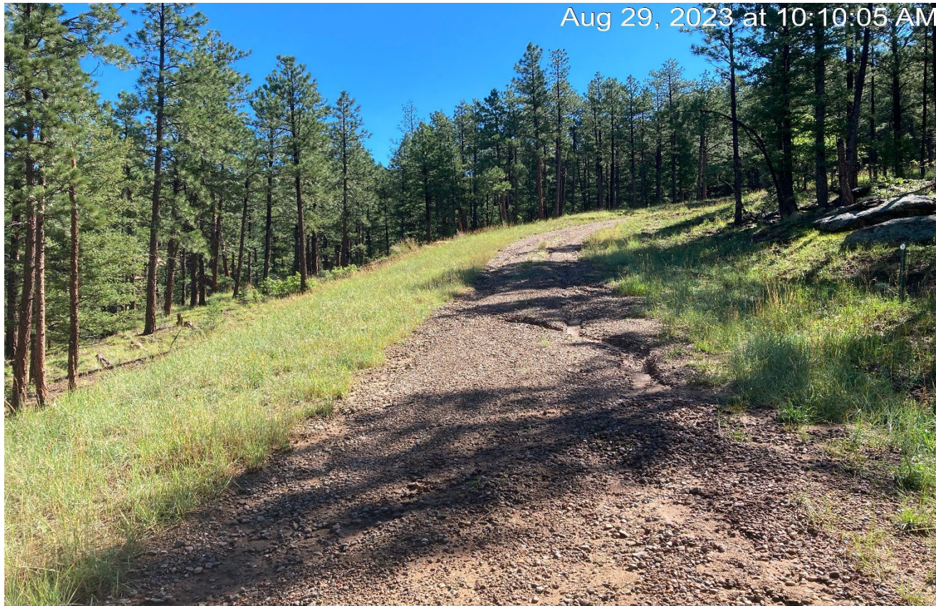
Photo 2. Facing northeast along the access road. Stormwater has washed down the access road causing erosion.
