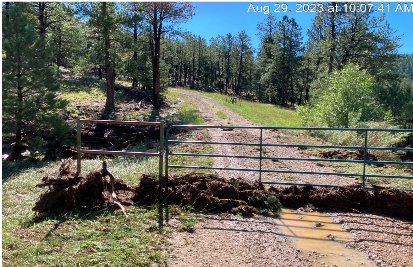
Photo 1. Facing east toward the access road. A recent heavy rainstorm has washed sediment and debris onto the road and gate.
