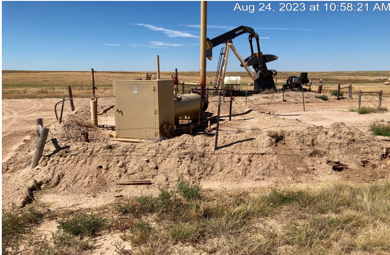
Photo 4. The south toward the wellsite and production equipment. The fence around the equipment is inadequate to prevent livestock entry. Cattle track have been observed inside the 2 strand fence.
