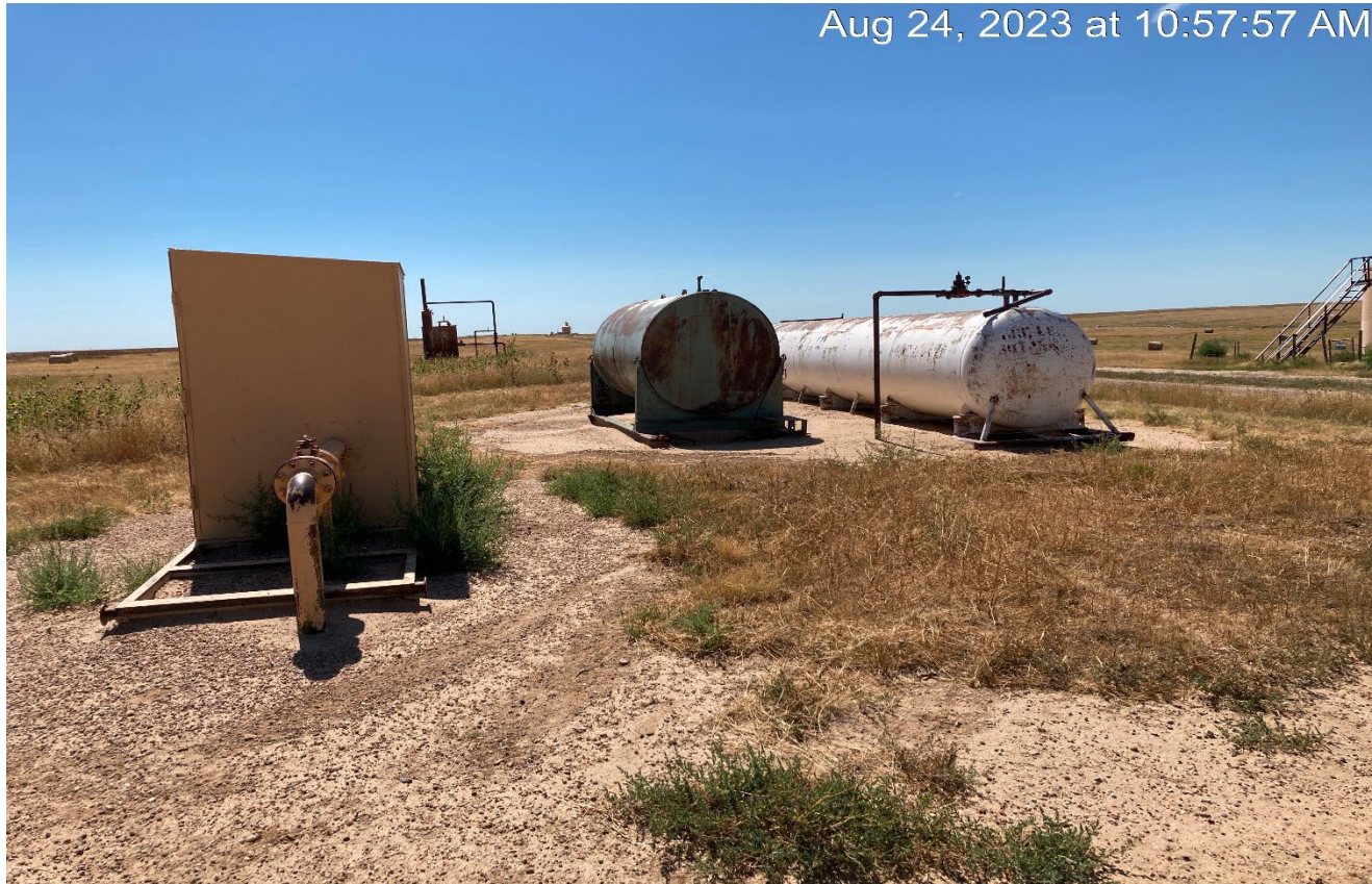
Photo 3. Facing southeast at the location. The two large volume tanks do not have proper labeling or secondary containment. If the tanks are unused then they need to be removed. Previous corrective action was not completed.
