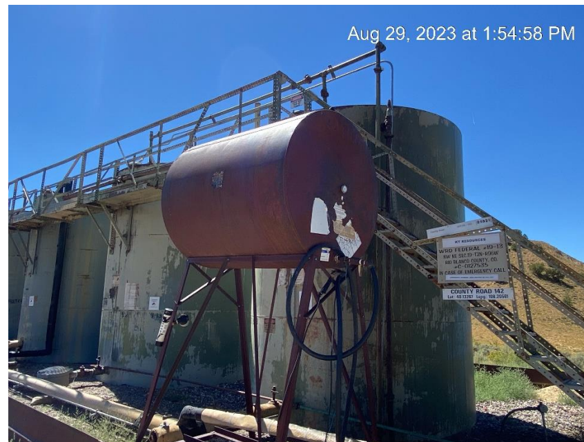
Unlabeled methanol tank
