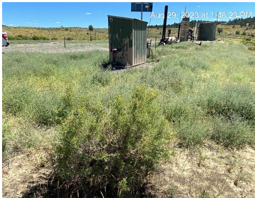
Location from Northwest corner. Weeds.
