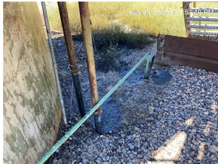
Leak? Large area covered in spray.
