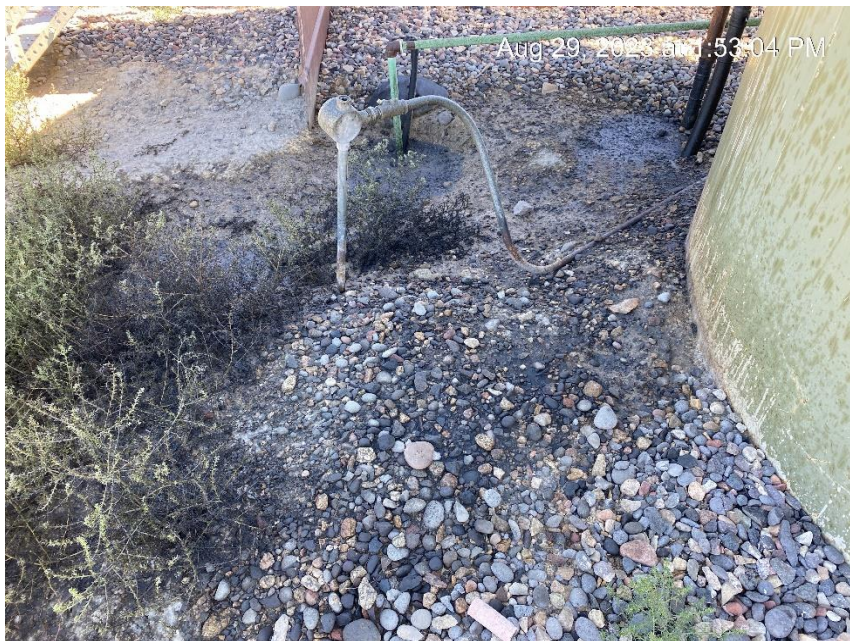
Leak? Large area covered in spray.
