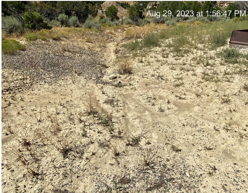
Insufficient Stormwater BMPs
