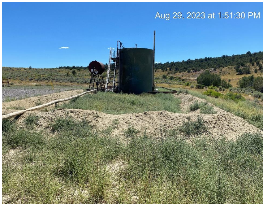
Weeds covering all of location
