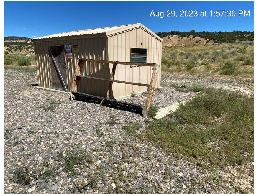
Debris still leaning against pump house. Weeds
