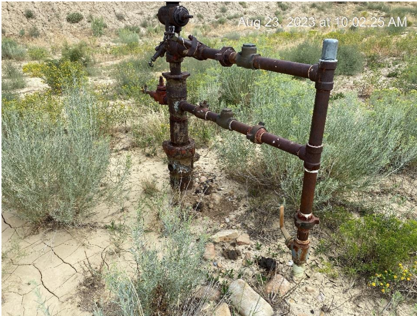
Venting. No valve in wellhead. Sediment migration.
