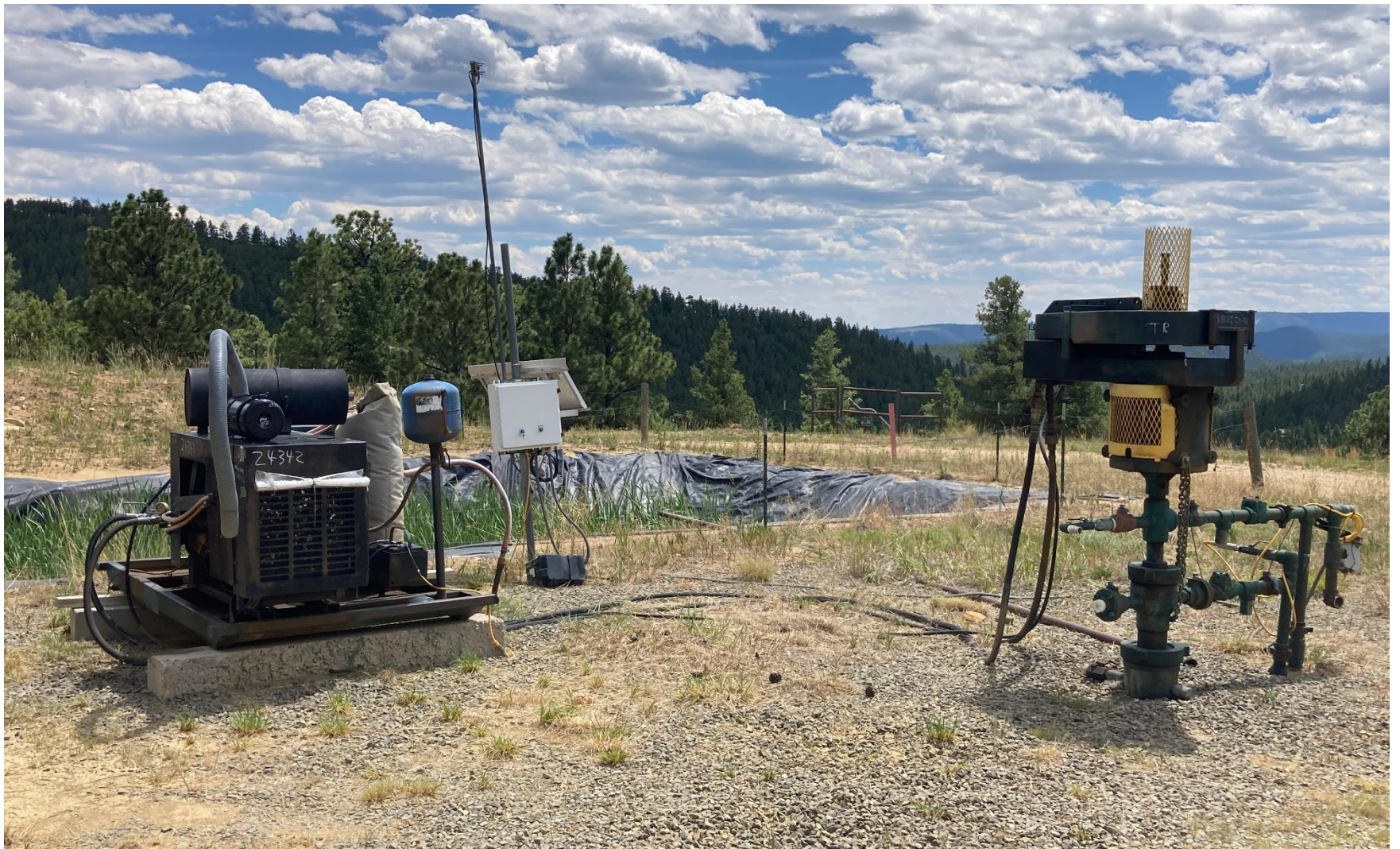
PHOTO 3: WELLHEAD AND EQUIPMENT
