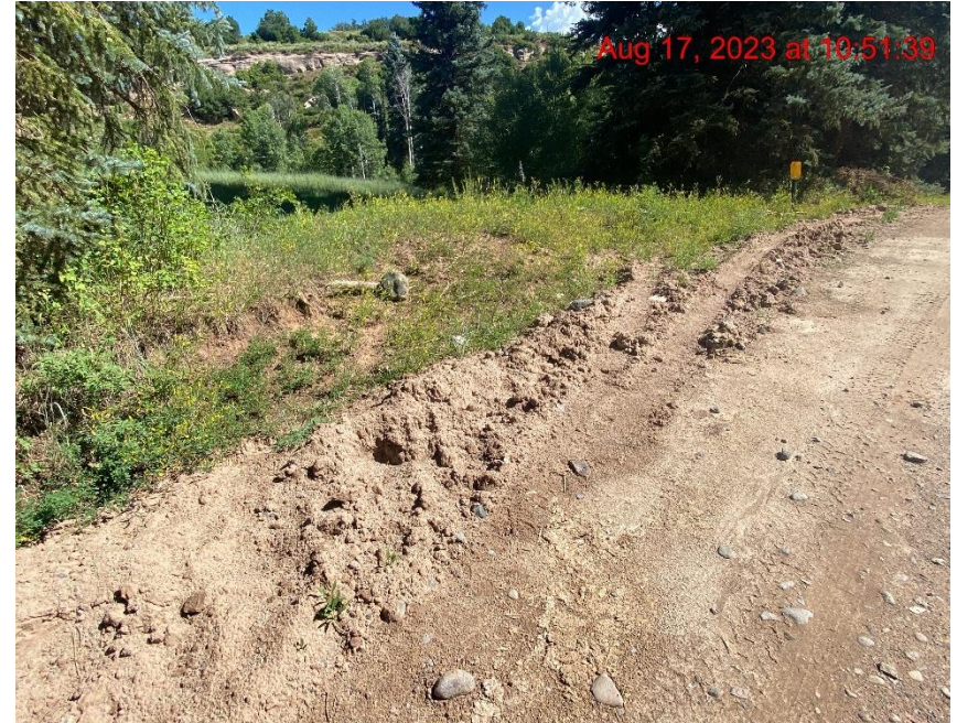
Lease Road Degradation at Clear Fork Crossing – Photo #05923
