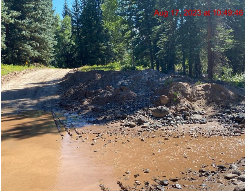
Unprotected Soil Stockpiles at Clear Fork Crossing – Photo #05917
