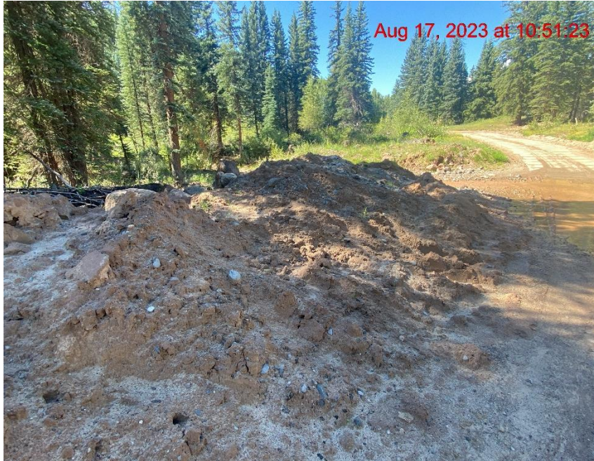
Unprotected Soil Stockpiles at Clear Fork Crossing – Photo #05921
