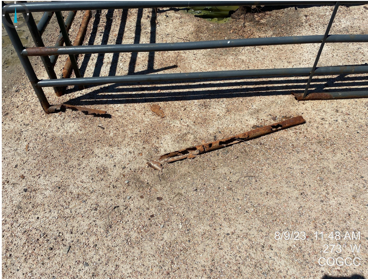
Photo 7. Debris from the location will need to be removed.
