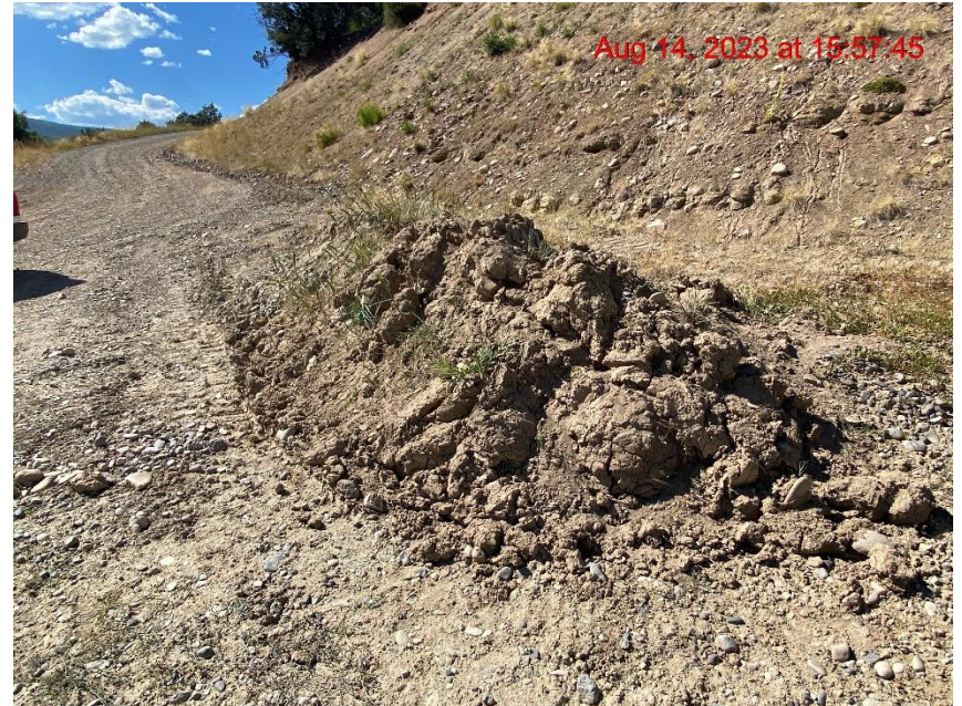
Unprotected Soil Stockpile – Photo #05884
