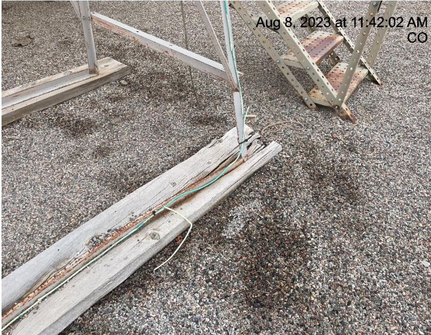
Photo # 5331 Stained gravel in secondary containment
