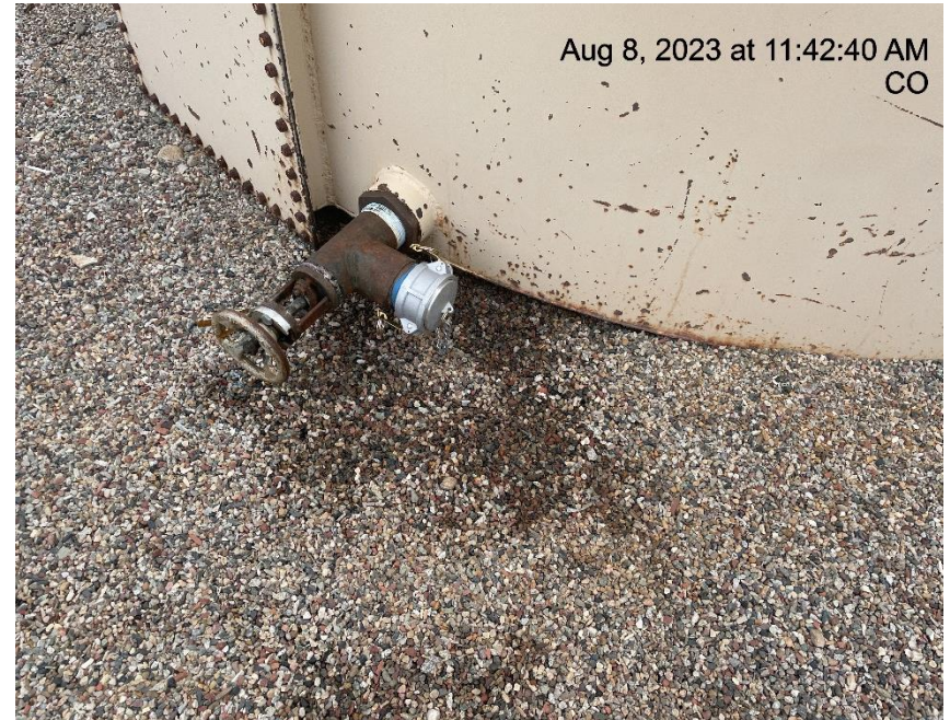
Photo # 5334 Stained gravel in secondary containment
