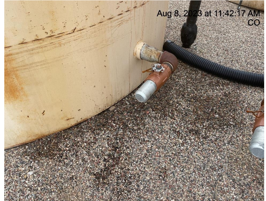
Photo # 5332 Stained gravel in secondary containment
