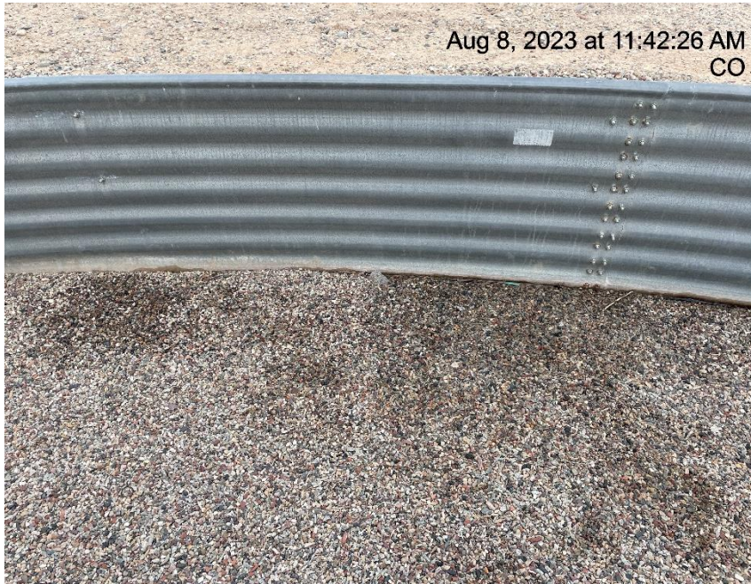
Photo # 5333 Stained gravel in secondary containment
