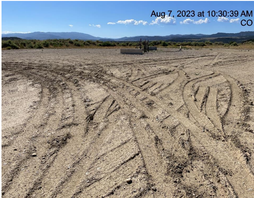
Photo # 4922 Lack of stabilization/compaction on location
