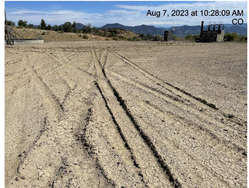
Photo # 4916 Lack of stabilization/compaction on location
