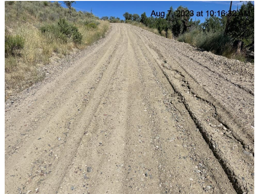
Photo # 4902 Erosion & transport of sediment on lease road
