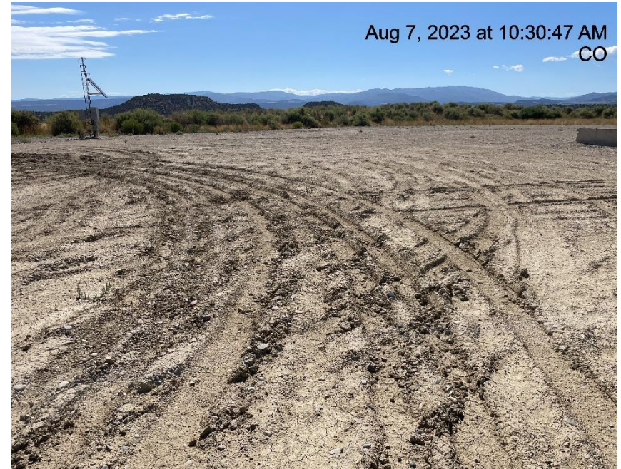
Photo # 4923 Lack of stabilization/compaction on location
