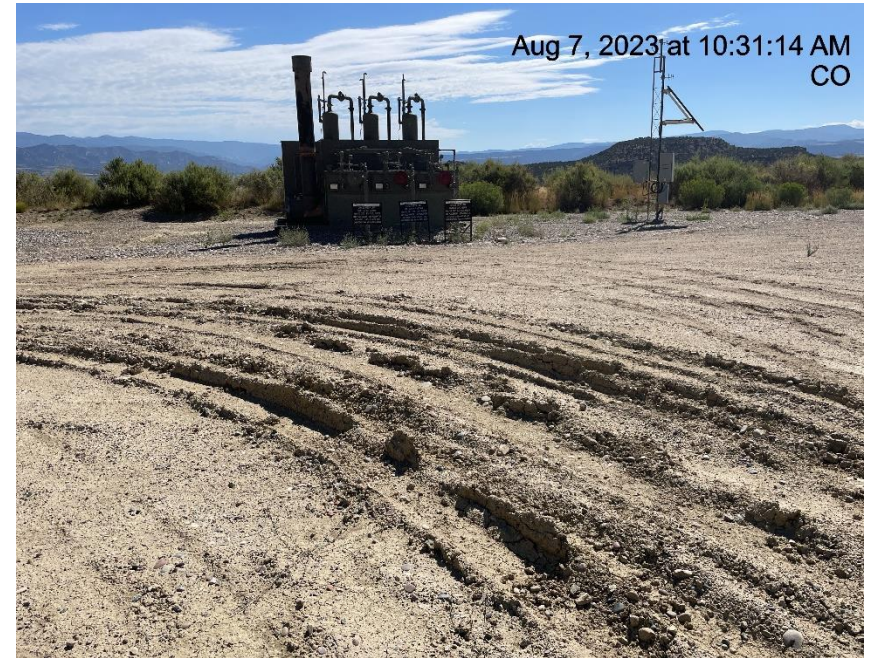
Photo # 4926 Lack of stabilization/compaction on location
