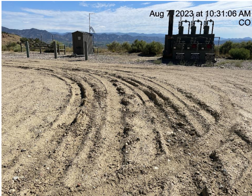
Photo # 4925 Lack of stabilization/compaction on location
