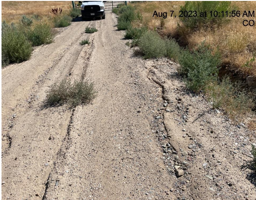
Photo # 4896 Erosion & transport of sediment on lease road
