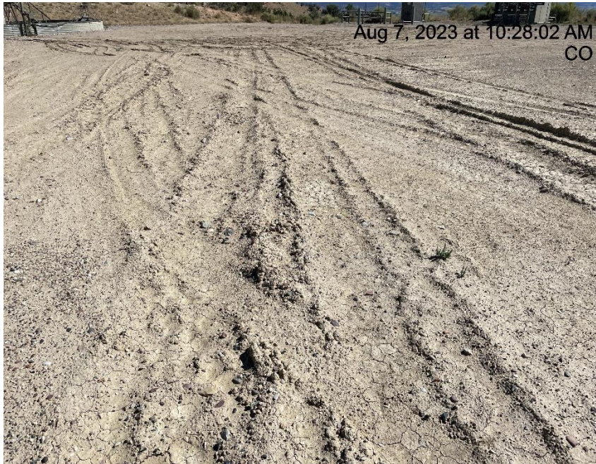
Photo # 4915 Lack of stabilization/compaction on location
