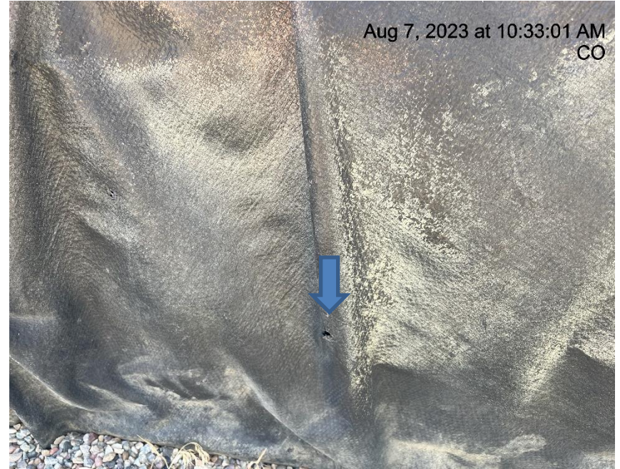
Photo # 5000 Secondary containment liner needs maintenance
