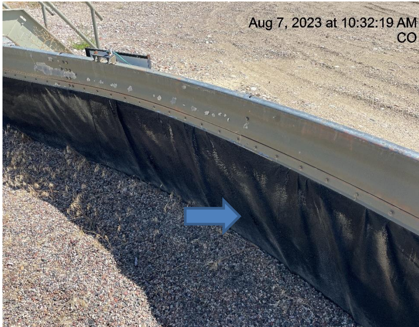
Photo # 4932 Secondary containment liner needs maintenance
