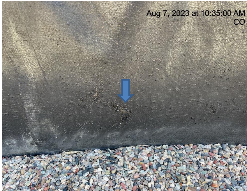
Photo # 4953 Secondary containment liner needs maintenance
