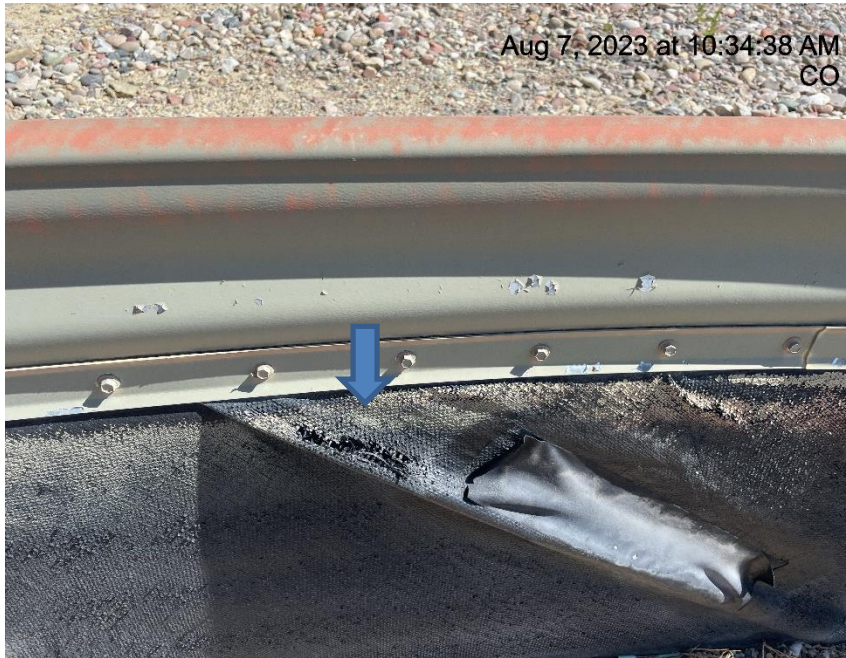
Photo # 4949 Secondary containment liner needs maintenance
