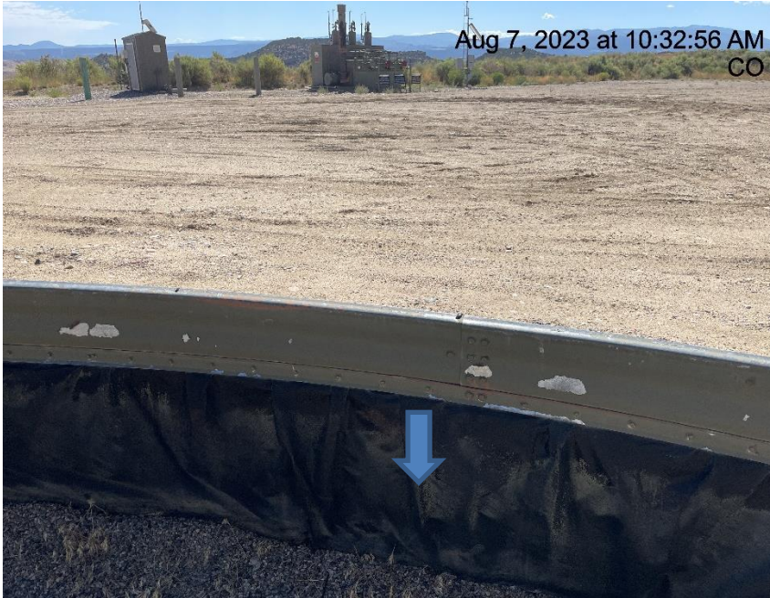
Photo # 4937 Secondary containment liner needs maintenance
