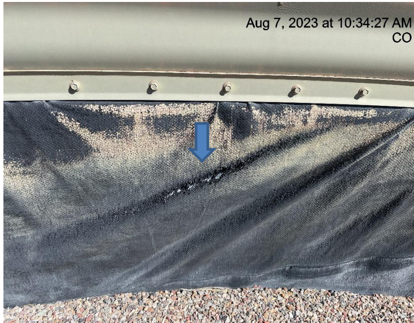
Photo # 4947 Secondary containment liner needs maintenance
