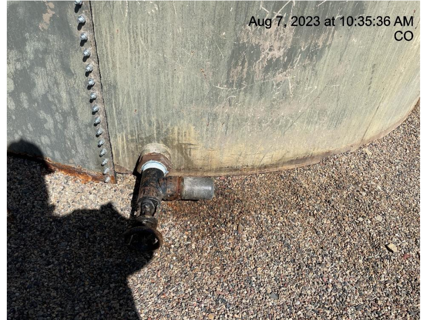
Photo # 4955 Stained gravel
