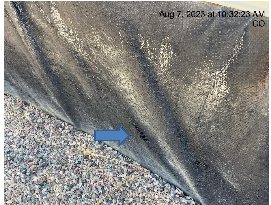
Photo # 4933 Secondary containment liner needs maintenance
