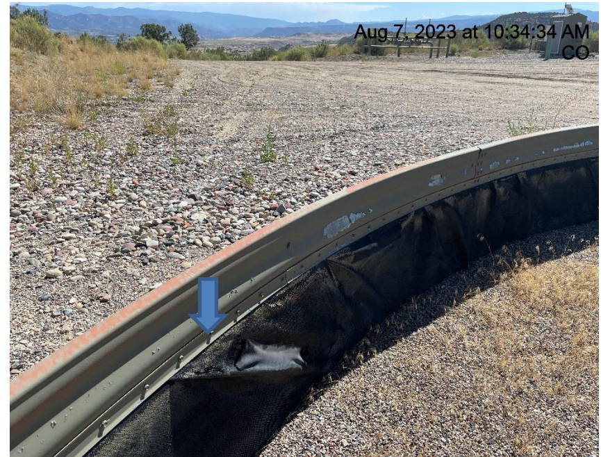
Photo # 4948 Secondary containment liner needs maintenance
