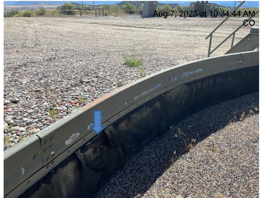
Photo # 5950 Secondary containment liner needs maintenance
