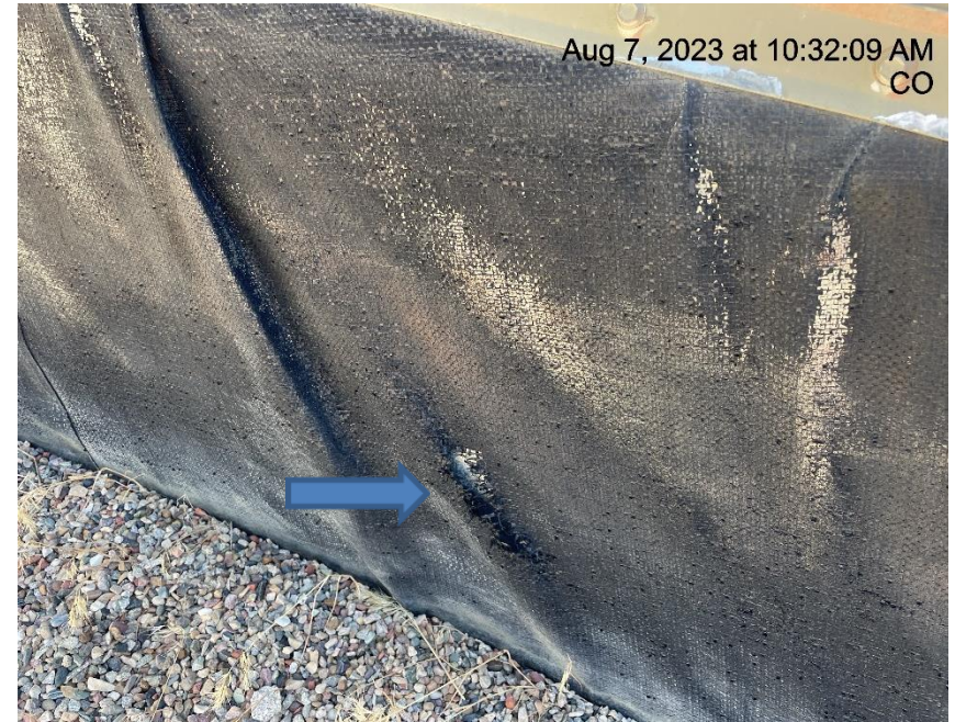
Photo # 4931 Secondary containment liner needs maintenance
