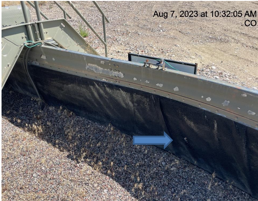
Photo # 4930 Secondary containment liner needs maintenance
