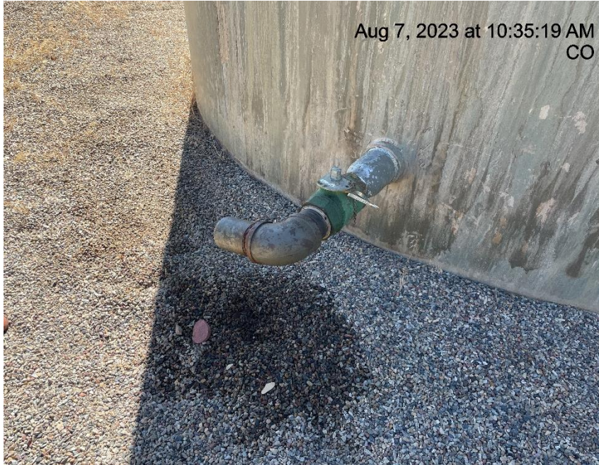
Photo # 4954 Stained gravel
