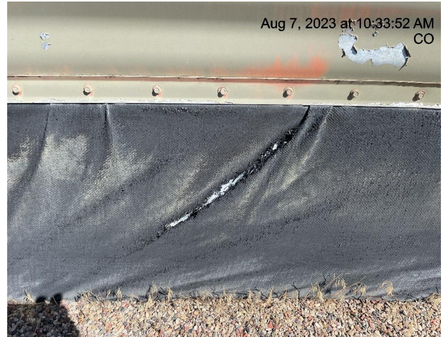
Photo # 4942 Secondary containment liner needs maintenance
