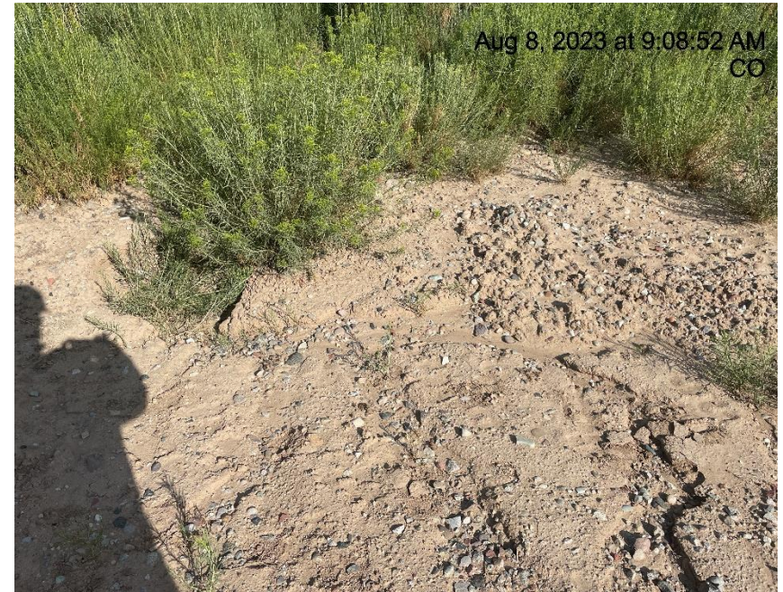
Photo # 5119 Erosion & transport of sediment (Near edge of pad near separator unit & Summit meter house)
