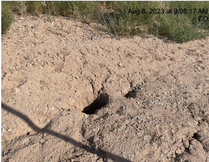
Photo # 5109 Tunnel erosion/sink hole (Edge of pad near separator unit & Summit meter house)
