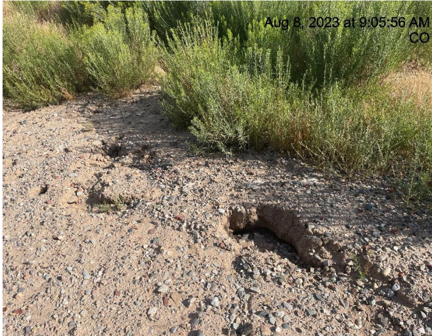
Photo # 5113 Tunnel erosion (Edge of pad near separator unit & Summit meter house)
