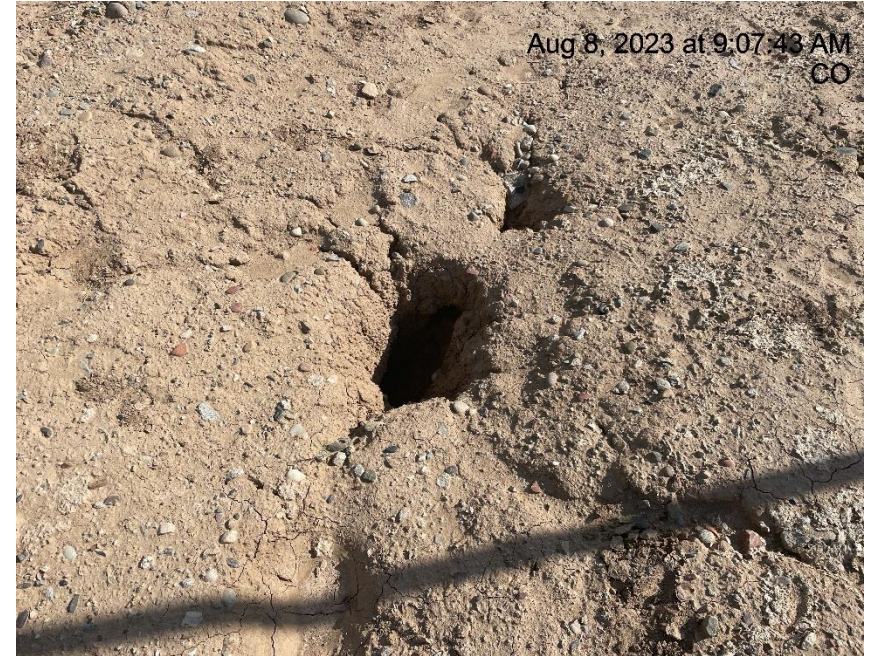
Photo # 5116 Tunnel erosion/sink hole (Near edge of pad near separator unit & Summit meter house)
