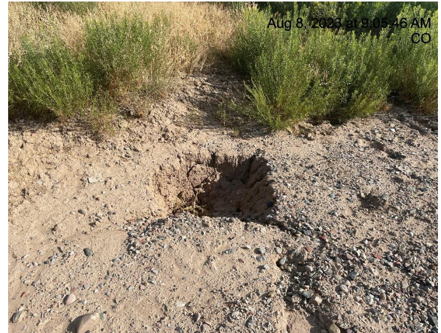
Photo # 5112 Tunnel erosion/sink hole (Edge of pad near separator unit & Summit meter house)
