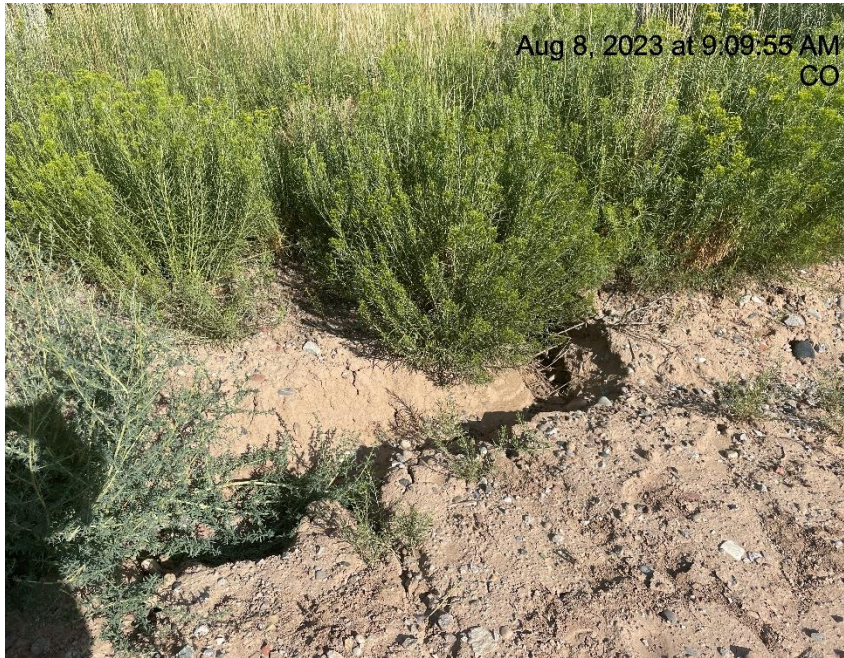
Photo # 5122 Erosion & transport of sediment off location into vegetation (west side of pad)
