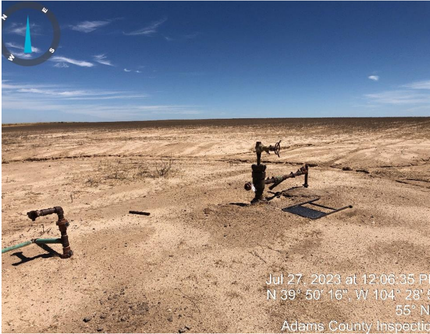
Photo #1 Well head.
