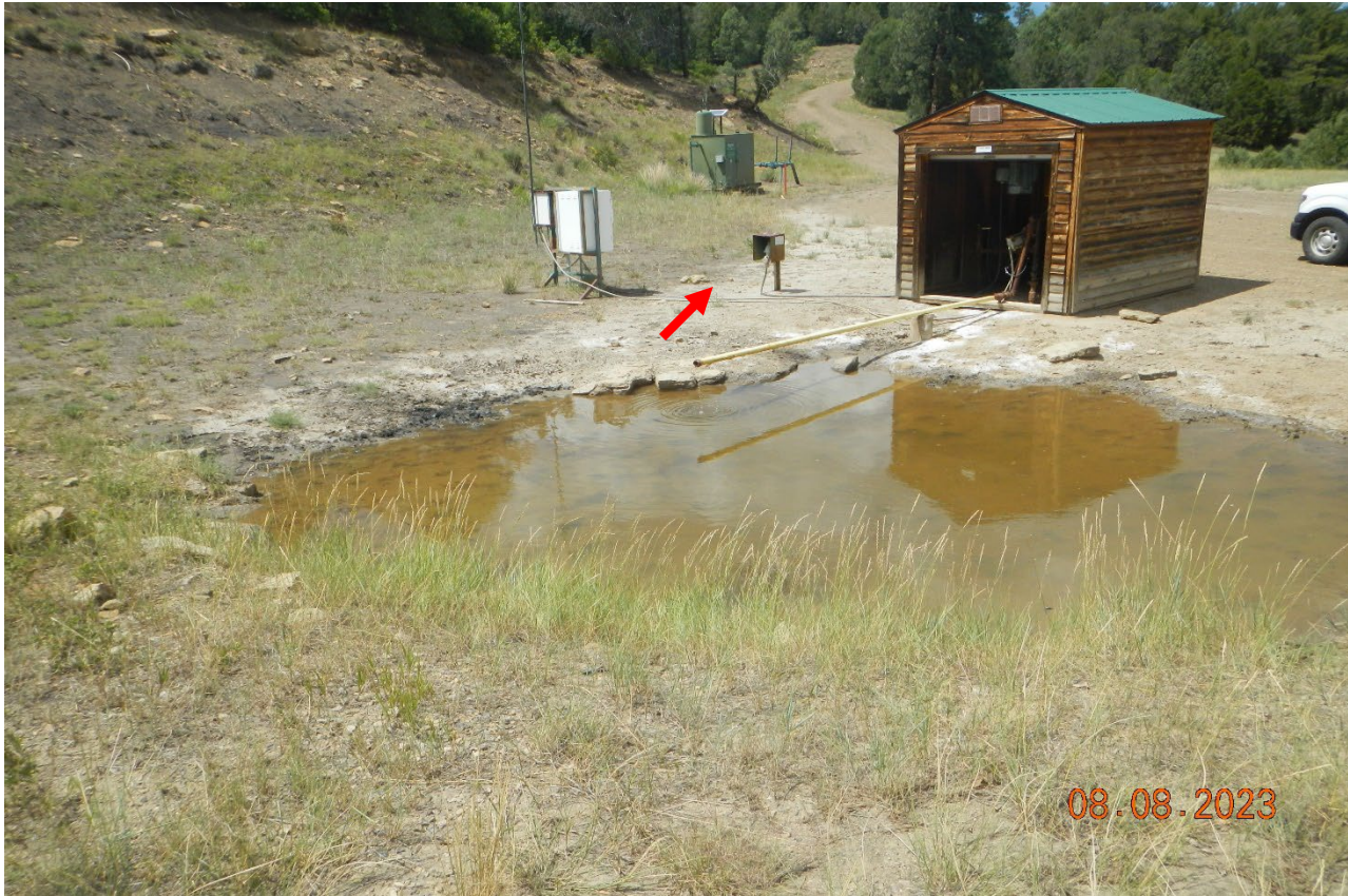
Photo 2. Facing toward the pit which is above freeboard level and is not constructed to allow adequate freeboard. There appears to be whitened soils where water may have over flowed toward the red arrow direction.
