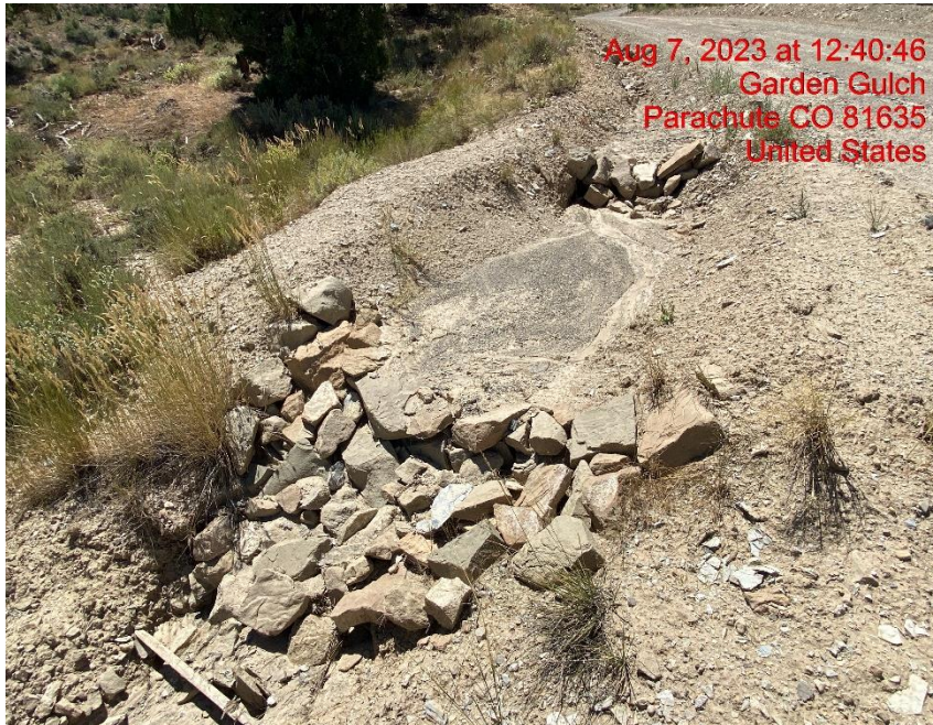
Check Dam Needs Maintenance – Photo #05611
