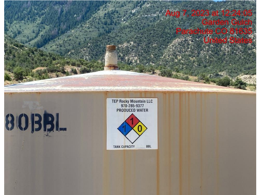
Tank Label Does Not State Capacity – Photo #05594
