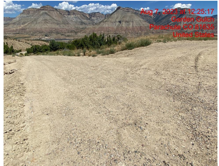
Insufficient Vehicle Tracking BMPs at Location Entrance/Exit – Photo #05598
