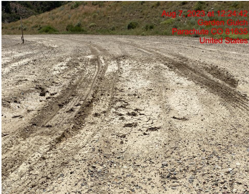
Location Lacks Stabilization – Photo #05596
