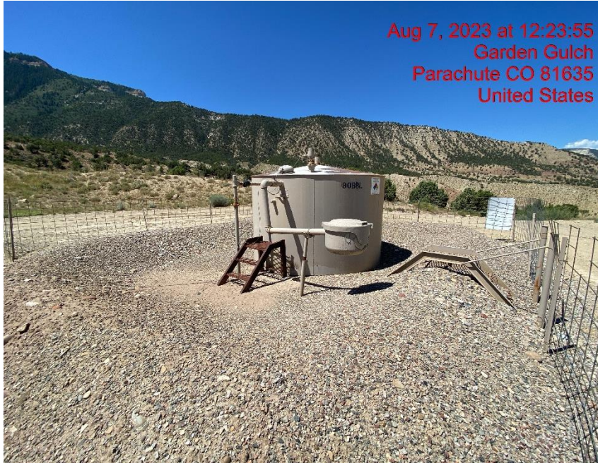
Tank Battery – Photo #05593
