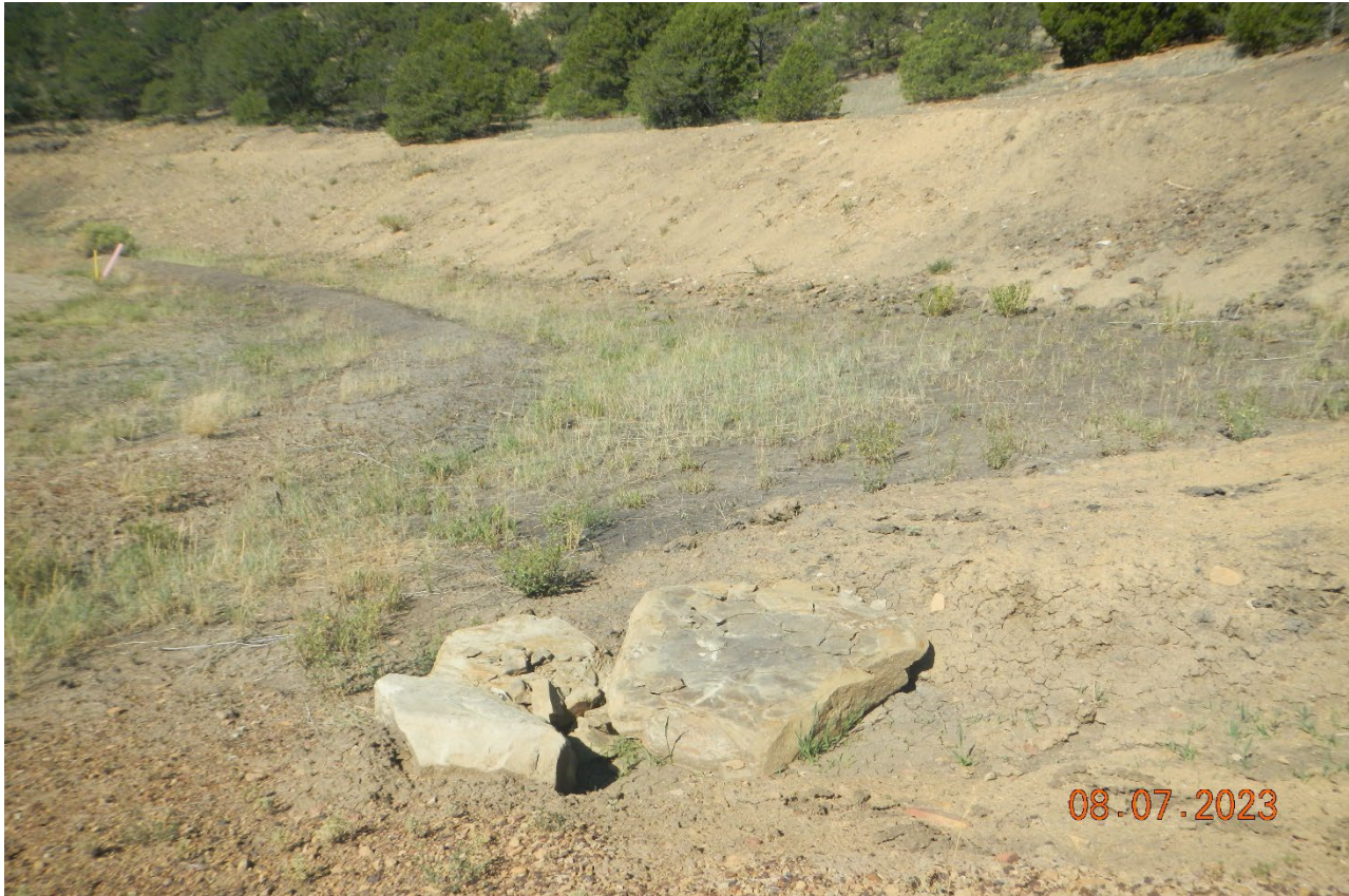
Photo 2. Facing toward the cut slope which has been repaired, seeded, and hydromulched.
