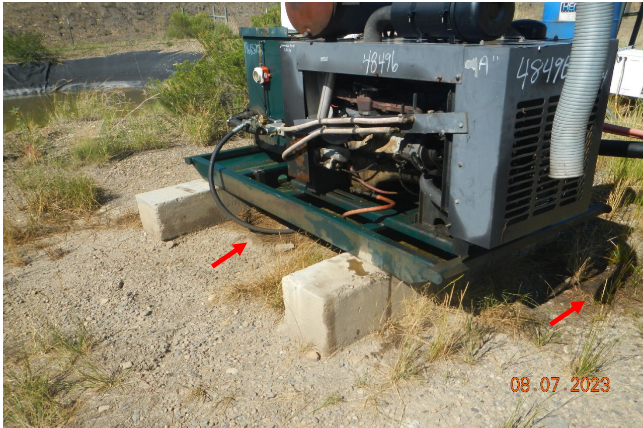
Photo 3. There is still oil stained soil around the engine skid .
