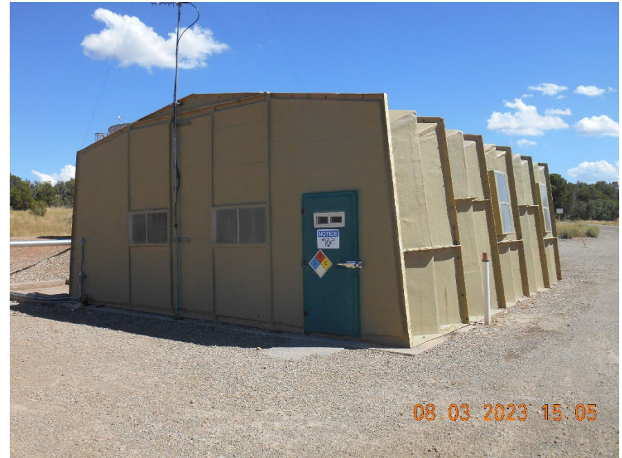
Manifold Housing and control station
