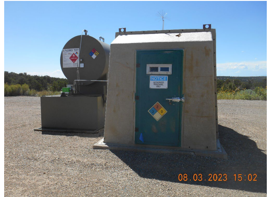
Injection wellhead housing Secondary containment of chemicals
