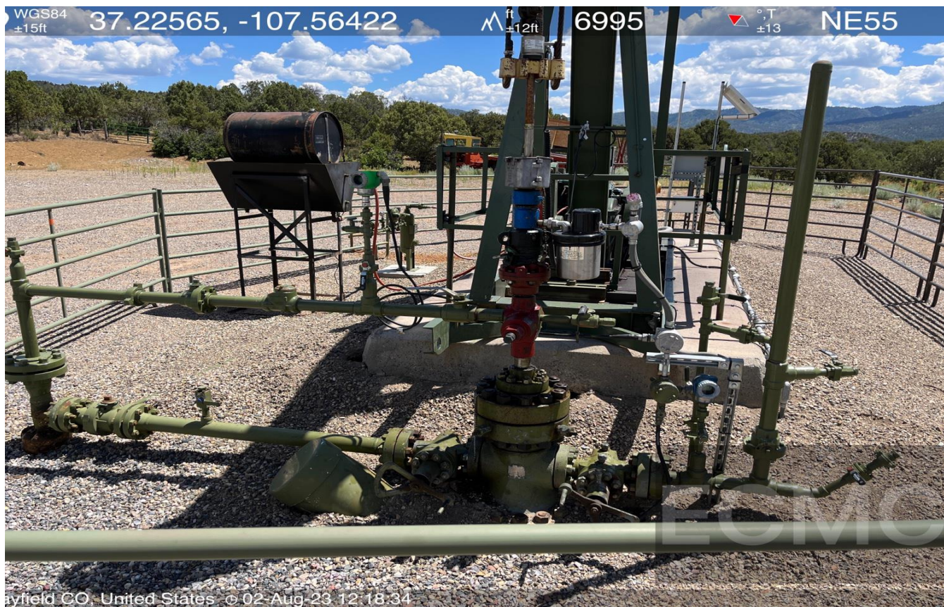
Photo #2. View of the wellhead assembly.
