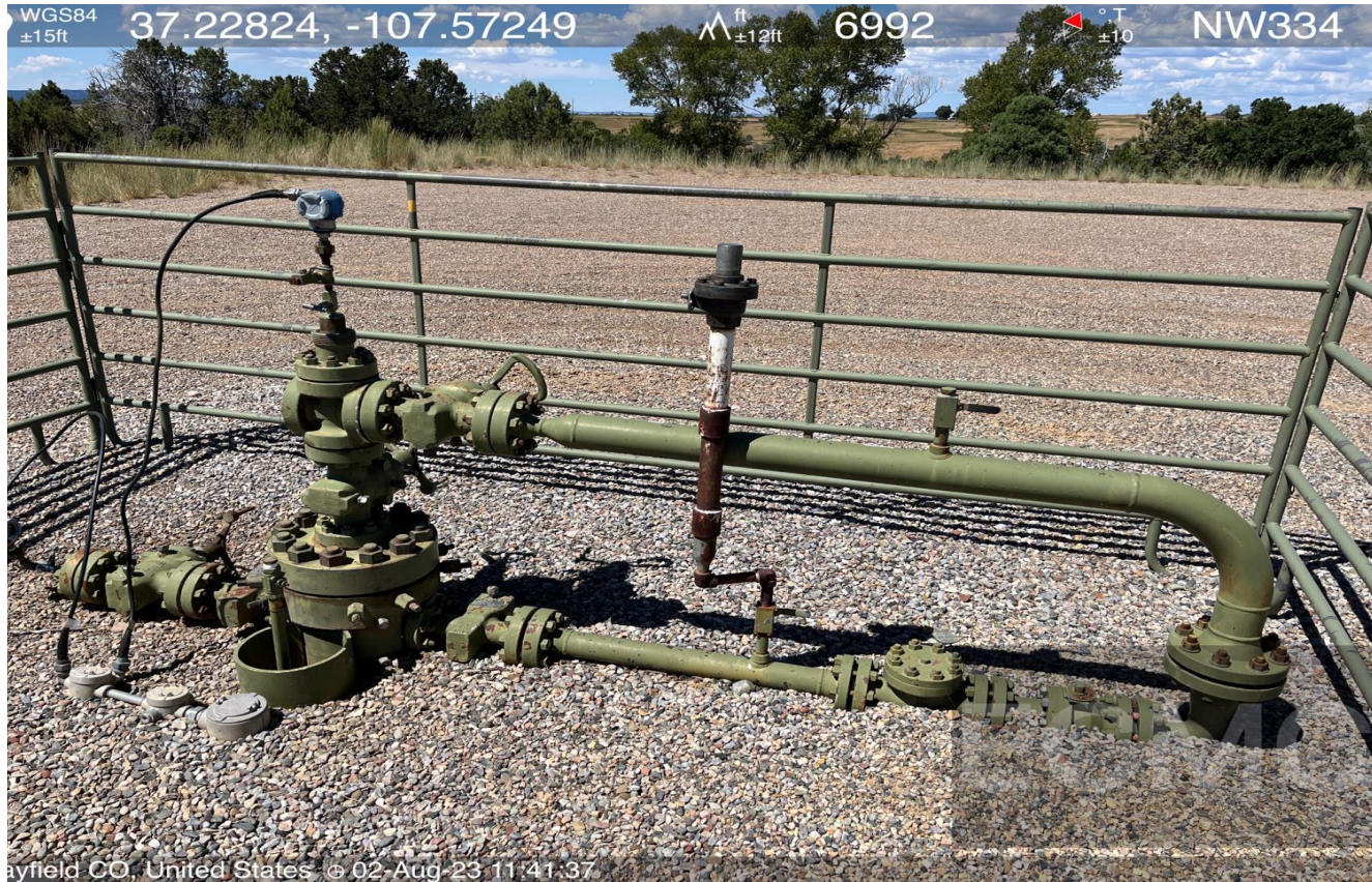
Photo #2. View of the wellhead assembly.
