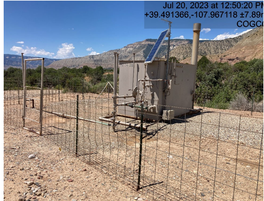
Separator and lack of meter calibration card access
