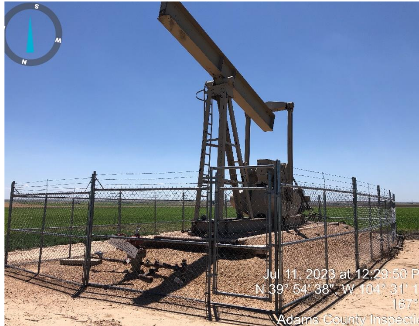
Photo# 13 T/A Pump jack.
