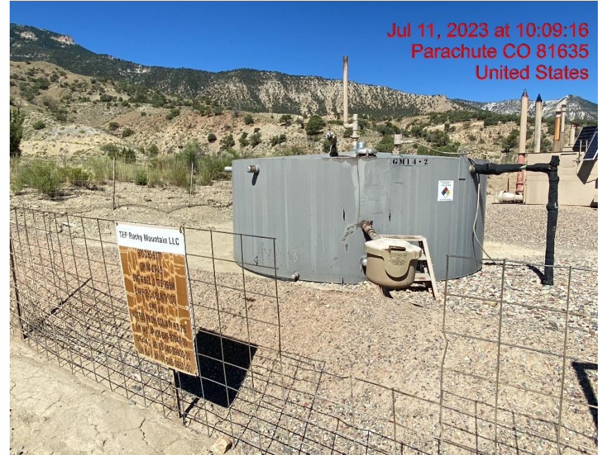
Tank Battery – Photo #05140
